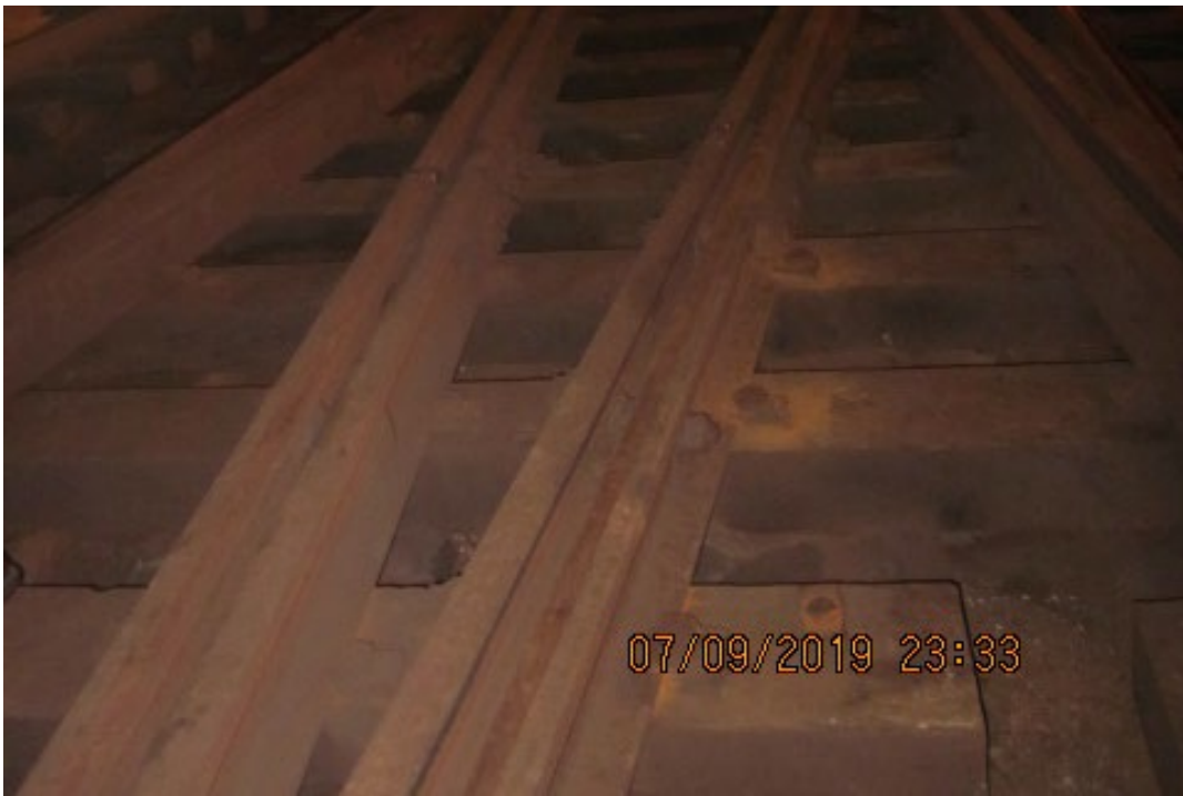
Figure 3 shows Local track 1 at Erie interlocking and the Type B track construction.
