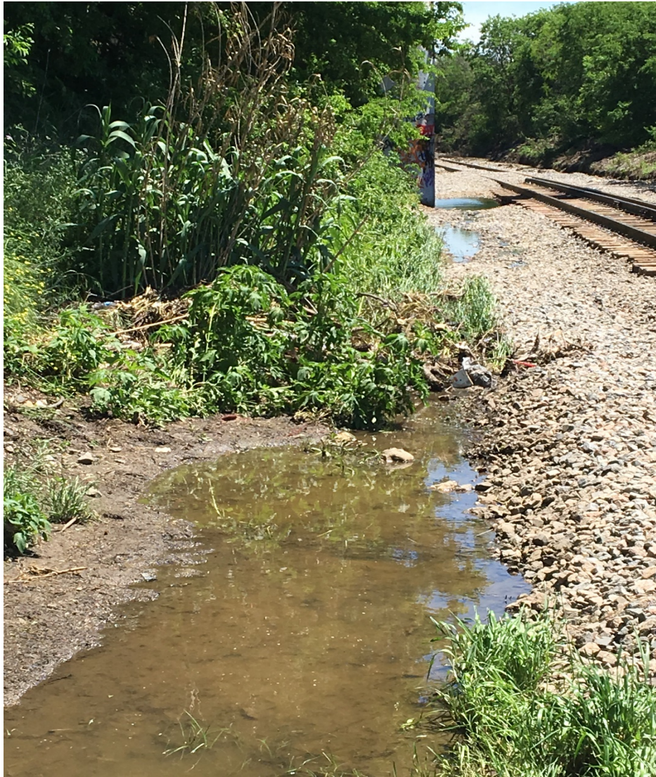
Figure 7- Photo taken from the left side (railroad east) of the track and looking south. Photo shows a standing pool of water from storm water run-off from the street drainage culvert, with tall vegetation laying over in a southward direction indication water flow direction. Note of east bridge abutment wall of the Fort Worth and Western Railroad overhead bridge.
