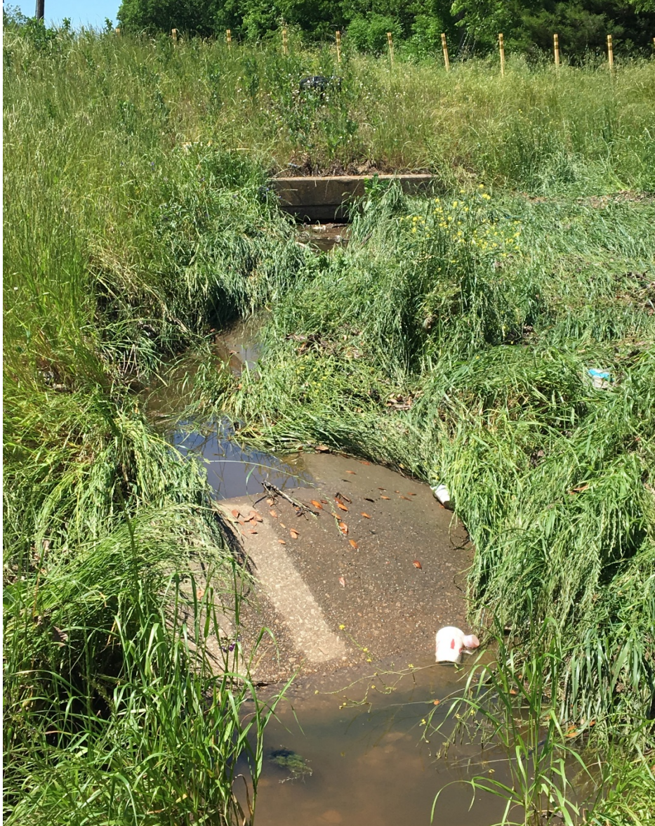
Figure 10- photo shows the Shamblee Drive street drainage culvert with standing non-flowing water due to vegetation clogging the waterway.
