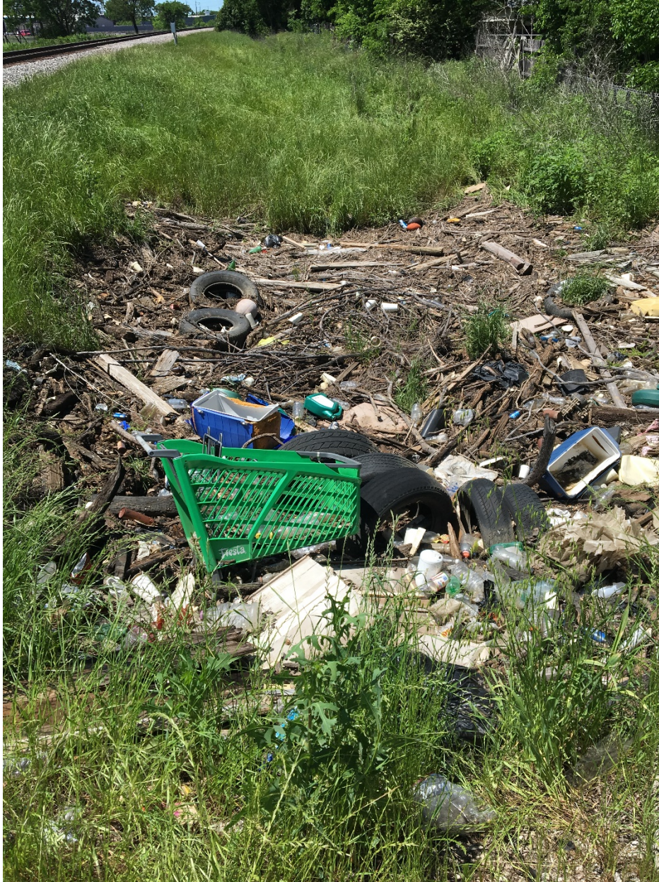
Figure 11- Photo is taken standing to the right side (railroad east) of the track and looking north. Photo shows a totally clogged drainage waterway with large amounts of trash, dirt and debris.
