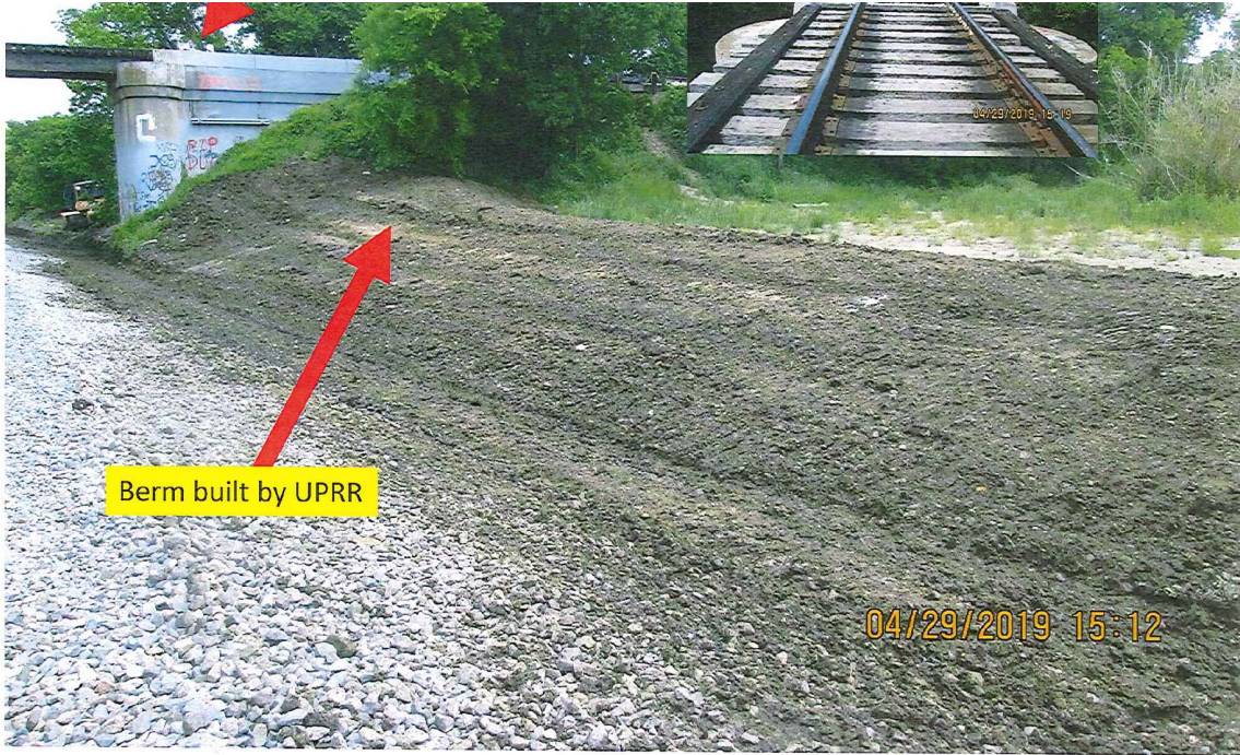
Figure 14- Photo shows a newly constructed water overflow berm constructed by Union Pacific to protect the railroad property from water overflowing from Lake Echo. (Photo courtesy of UP)
