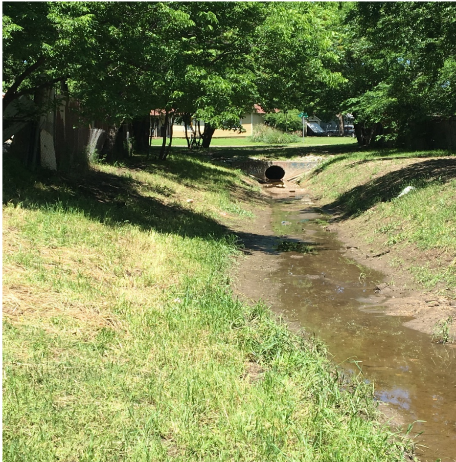
Figure 6- photo show a street drainage culvert located on the left side (railroad east) of the railroad with active water flowing onto the railroad property.
