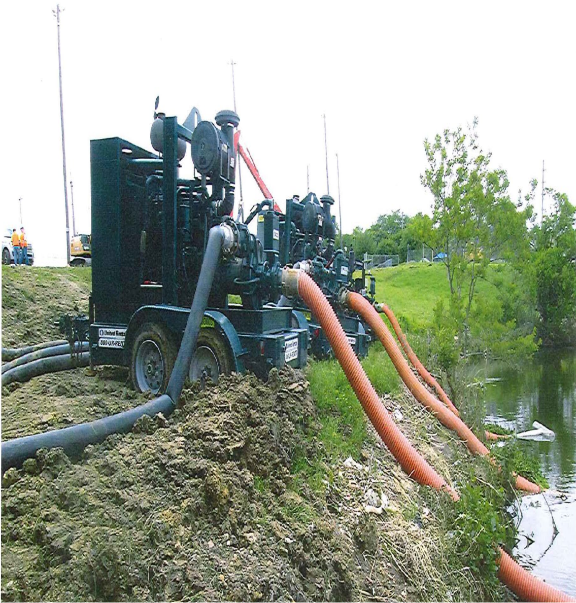
Figure 12- Large high-volume portable water pumps are being used to assist with lowering the water level in Lake Echo for lake culvert repairs. (Photo courtesy of UP)
