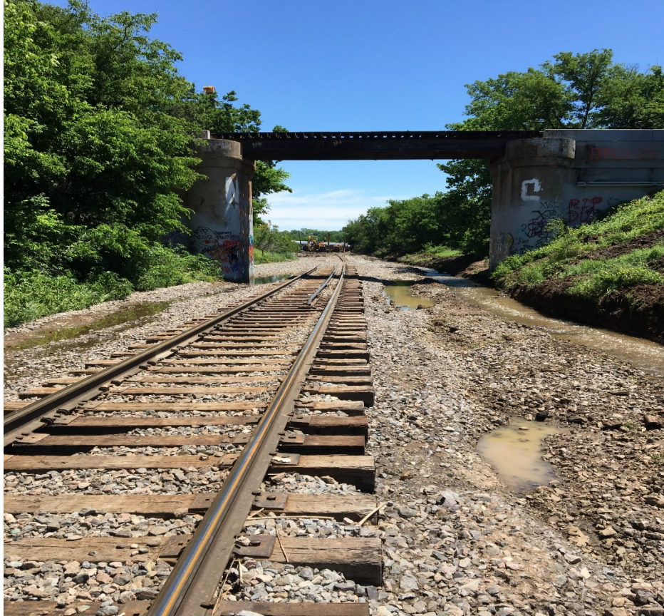
Figure 3- Post flooding and accident photo taken of the railroad track looking south towards the derailment location with active water flowing to the right (railroad west) and washed out shoulder and crib ballast. Note in the foreground where the ballast was washed up and over the railroad track.
