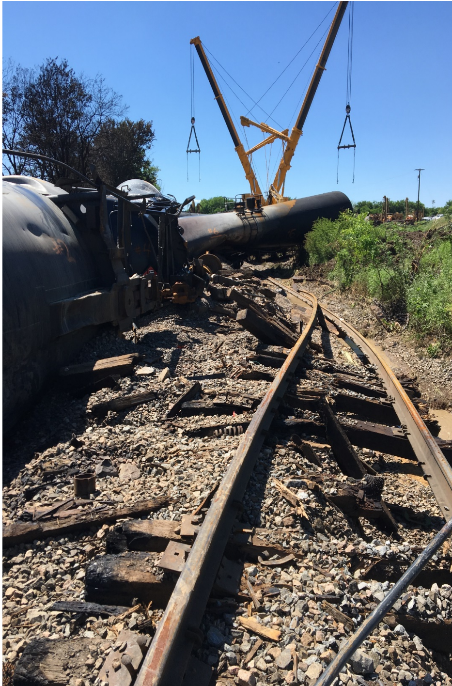
Figure 1- photo shows the destroyed track infrastructure and derailed/damaged tank cars with re-rail cranes working in the background. Picture is taken looking north in the area of the point of derailment at milepost 48.8.
