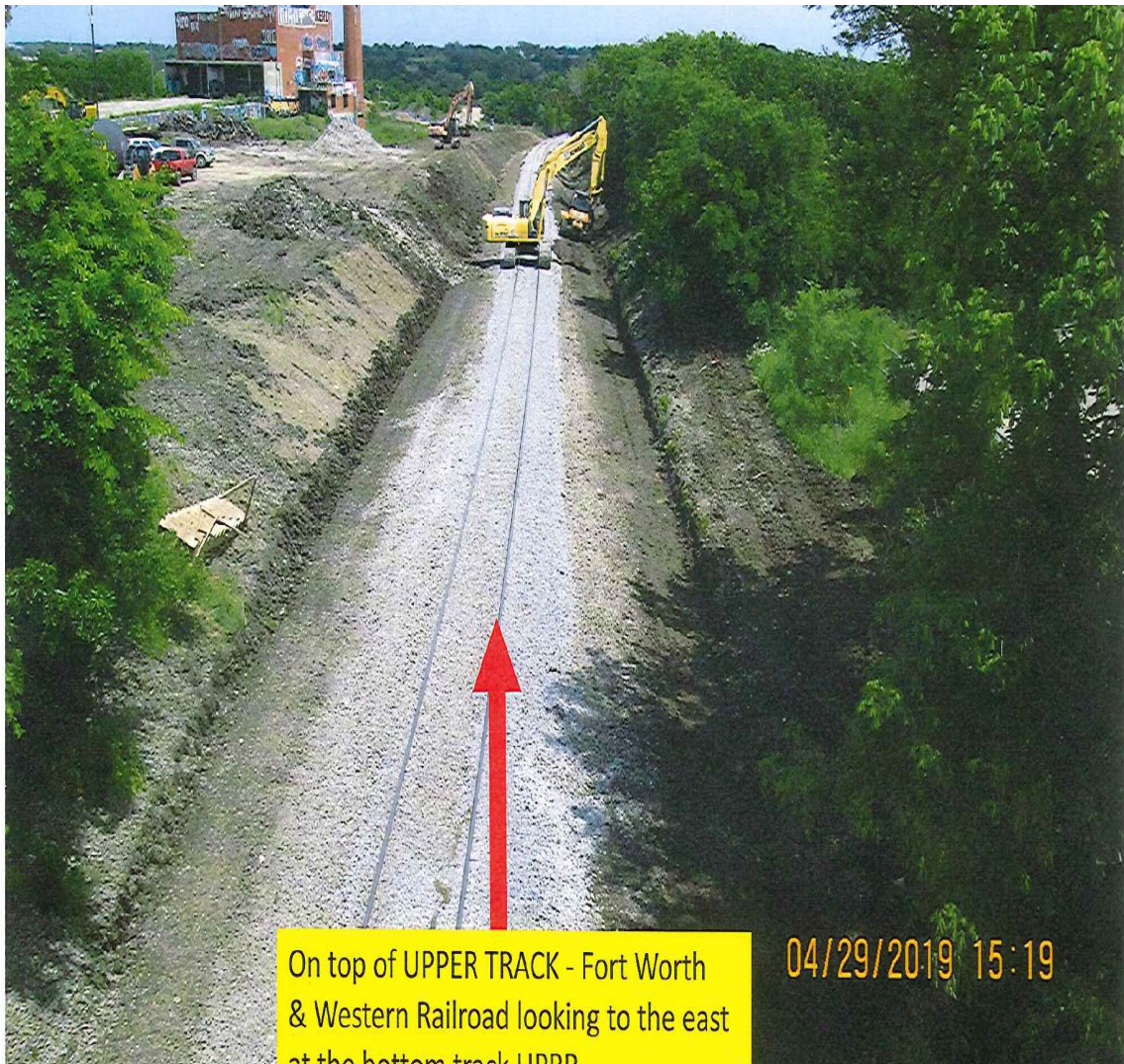
Figure 13- Overhead photo taken from the Fort Worth and Western Railroad overhead bridge showing the newly constructed track and new clean ballast looking south. The derailment occurred at the top portion of the photo where the track curves to the right. Note the track how digging the new west side drainage ditch and overflow berm. (Photo courtesy of UP)
