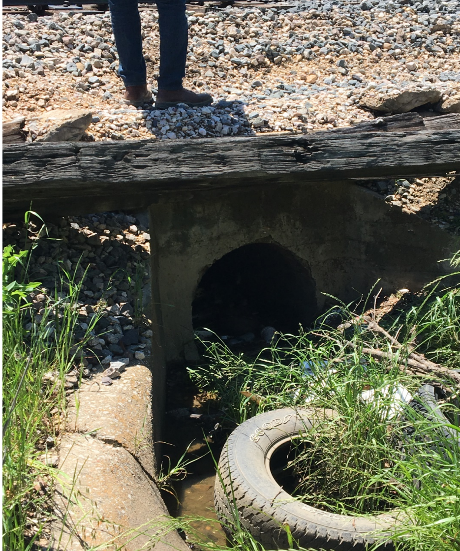
Figure 9- photo show a street drainage culvert that runs under the track and directs storm water run-off towards Echo Lake. Photo shows the drainage swell clogged and littered with trash, vegetation and debris.
