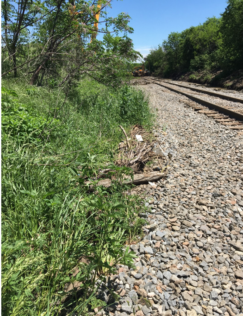
Figure 8- photo was taken while standing on the left side (railroad east) of the track and looking south. Picture shows vegetation laying over in a southward direction with debris piled up from the flow of storm water.
