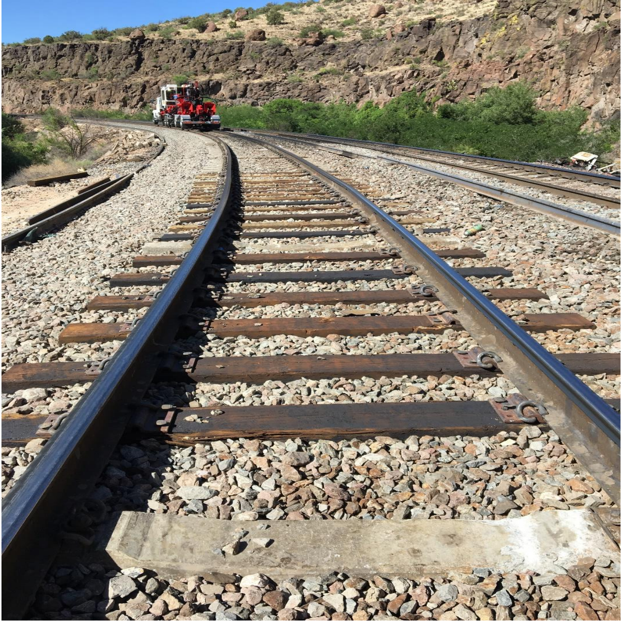
Figure 8. Picture looking eastward into curve #480A or collision site with an exemplar RUM.
