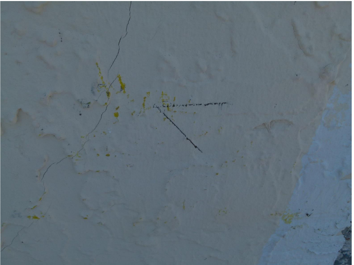
Figure 7: Angle drawn to paint transfer adjacent to 16G opening and window.
