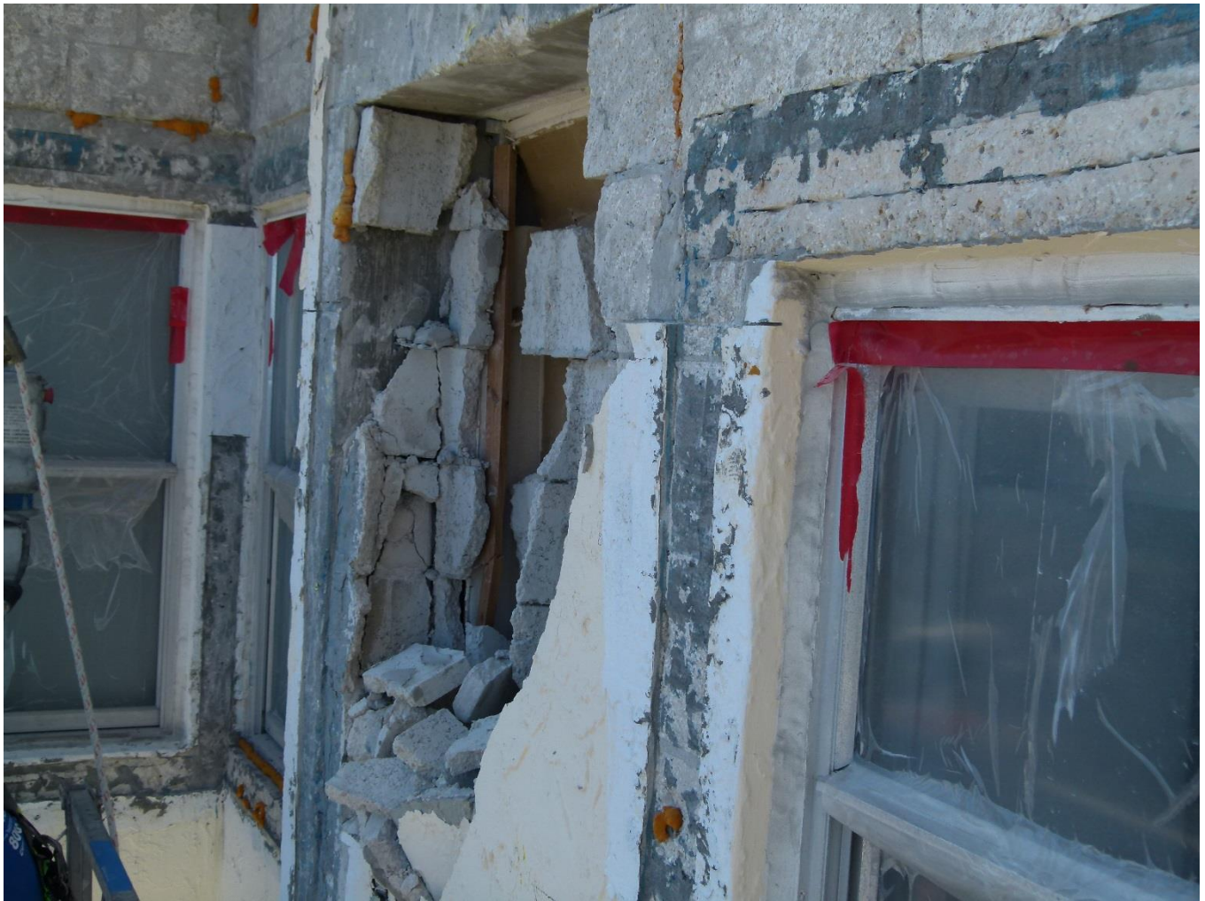
Figure 6: Opening in 16G showing damage and paint transfer markings.
