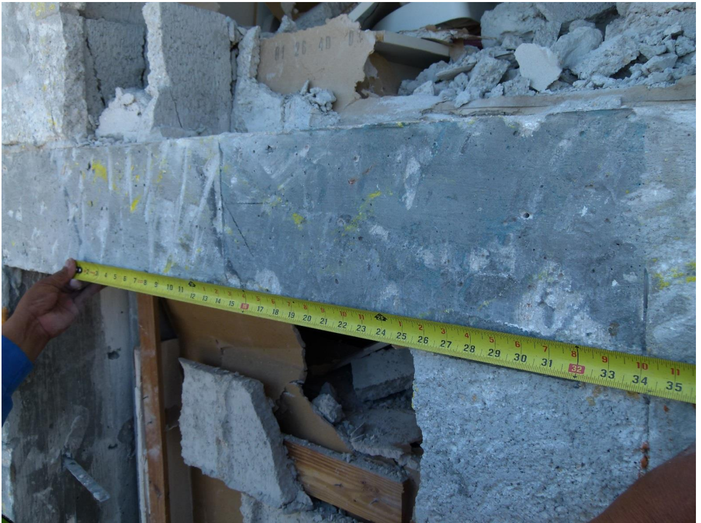
Figure 4: Vertical striations in concrete slab between 16G and 17 G.
