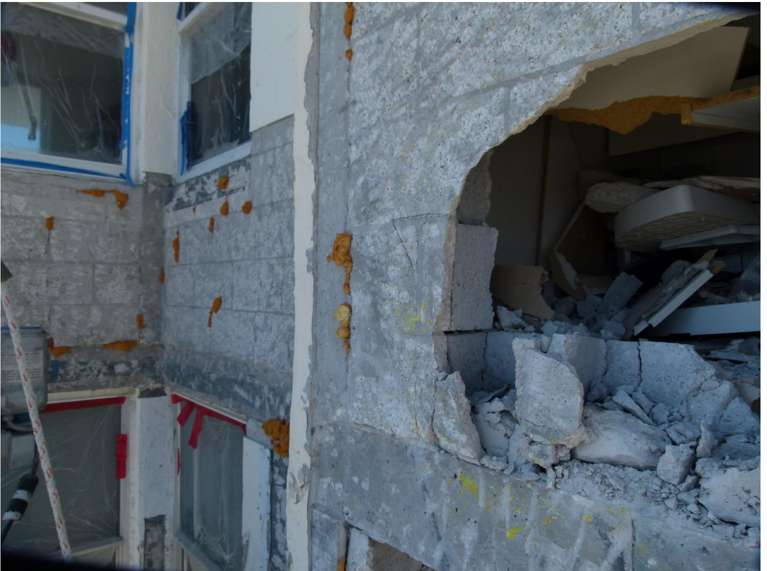
Figure 1: Opening in 17G showing damage and paint transfer markings.
