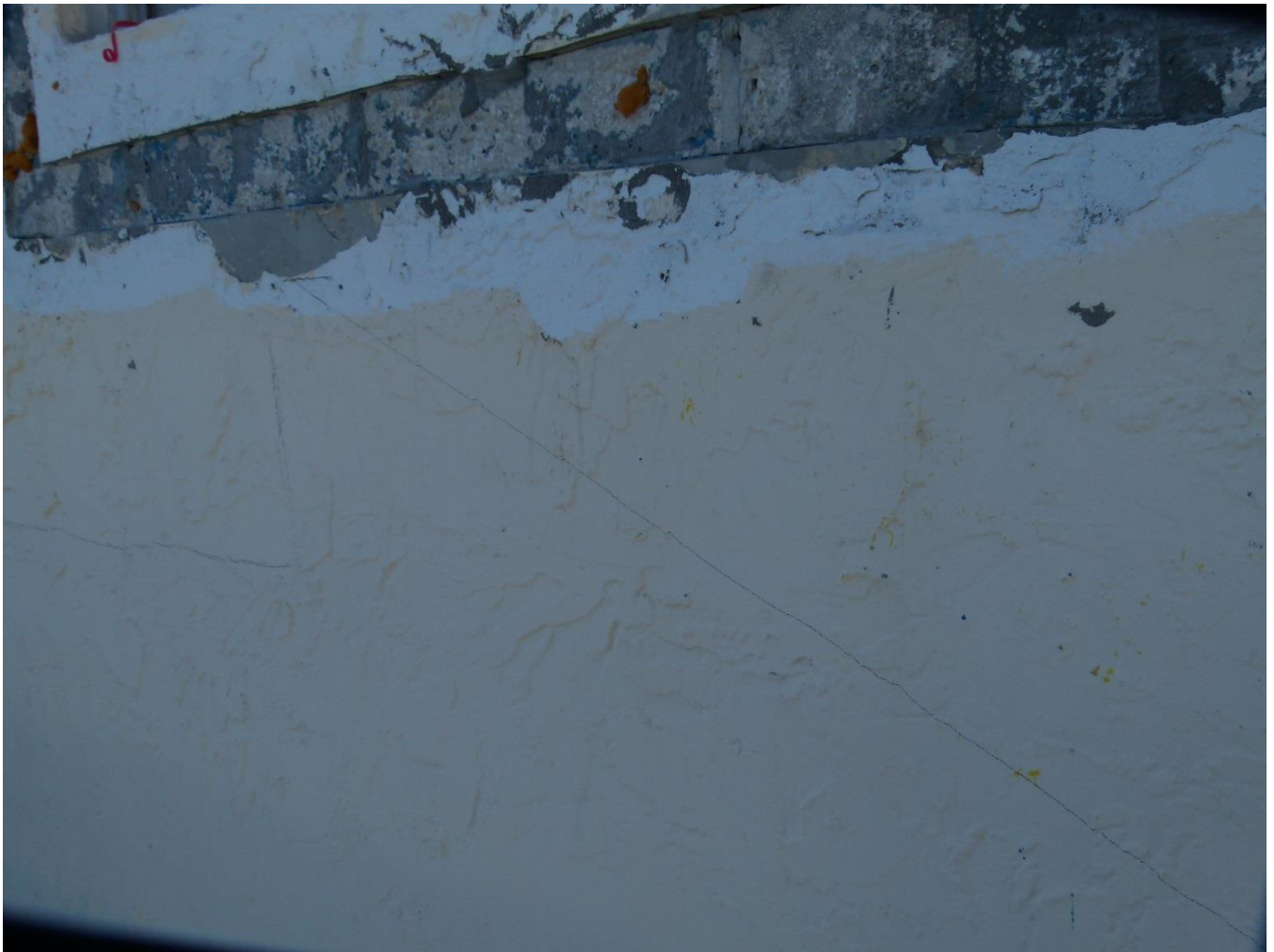
Figure 9: Paint transfer observed below and to the right of the window of 16G (adjacent to opening) angled downward towards unit 15F window with approx. angle drawn.
