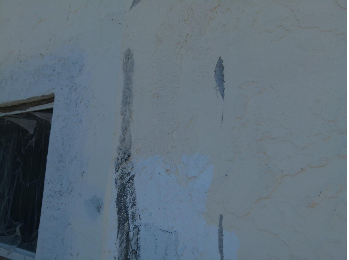
Figure 12: Paint transfer observed at unit 9G continuing downward along wall edge.
