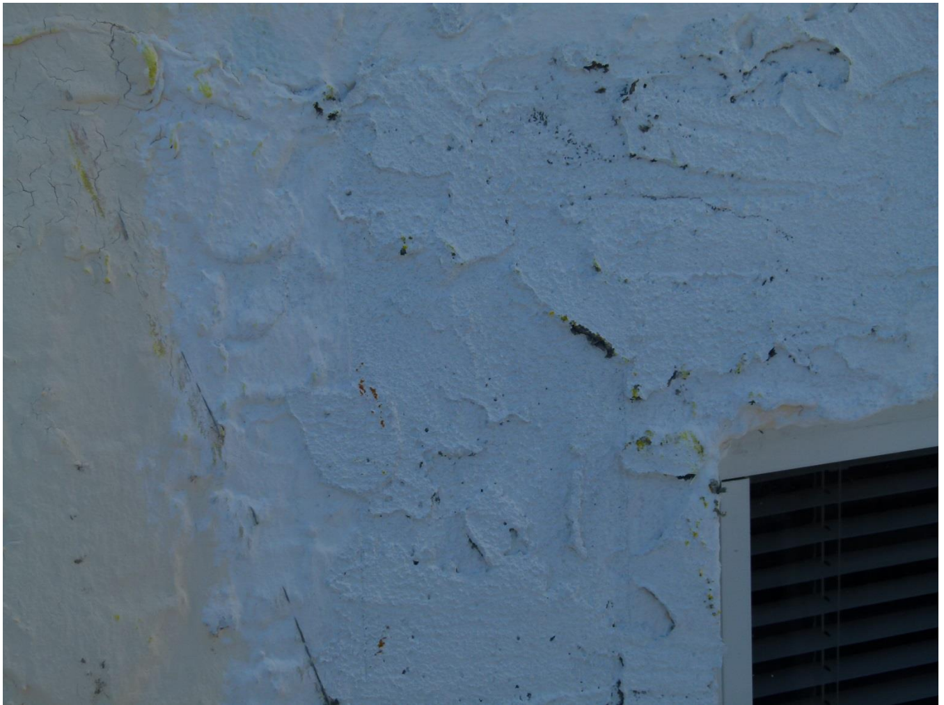
Figure 11: Paint transfer observed at 15G continuing downward along wall edge.
