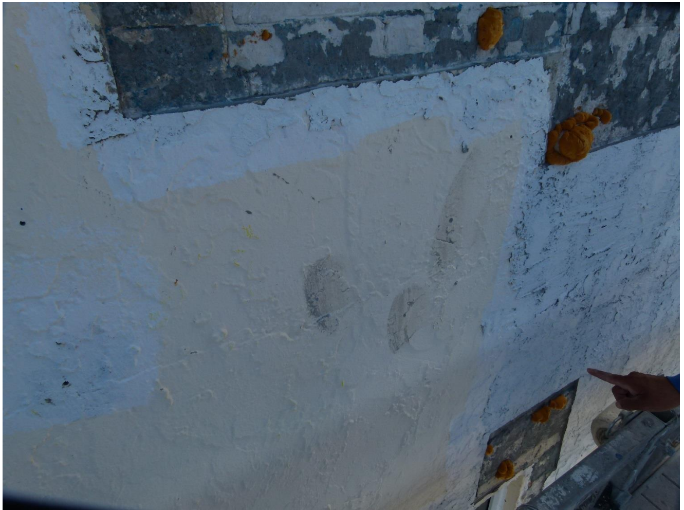
Figure 10: Paint transfer observed at unit 16F window, continuing downward on wall between units 15G and 15F
