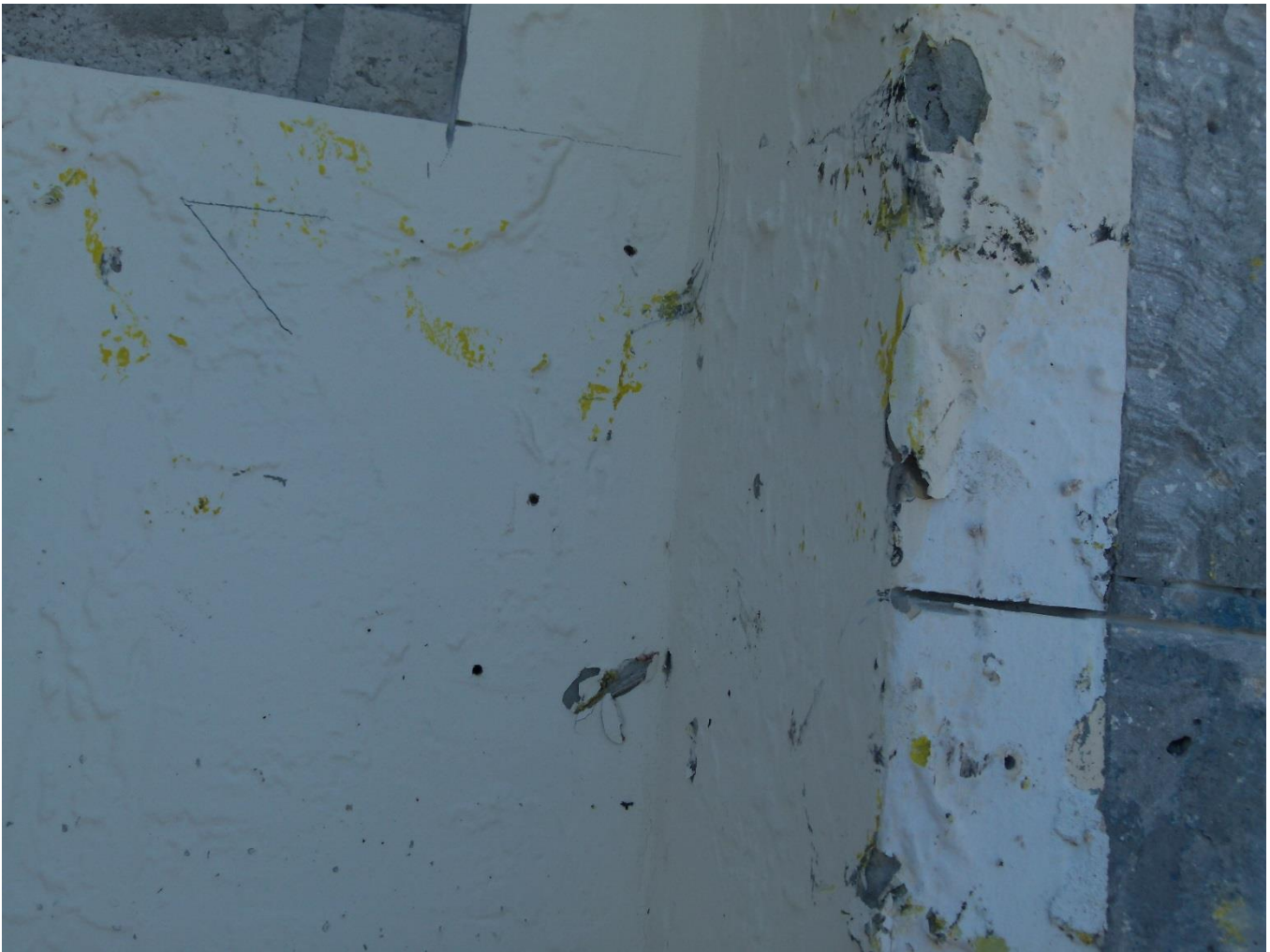
Figure 8: Stucco striations and paint transfer observed on south window stack wall of 16G (adjacent to opening) angled downward with approx. drawn angle.
