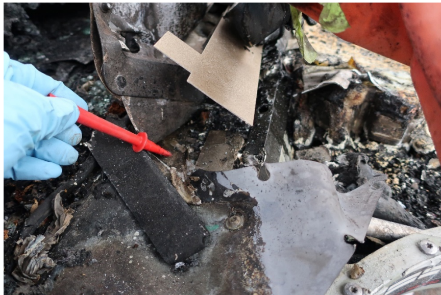
Figure 23. Top of module 13 after cleaning away fire debris, pointing at broken mica on plastic tray. The mica and plastic were able to be moved to see the cell
