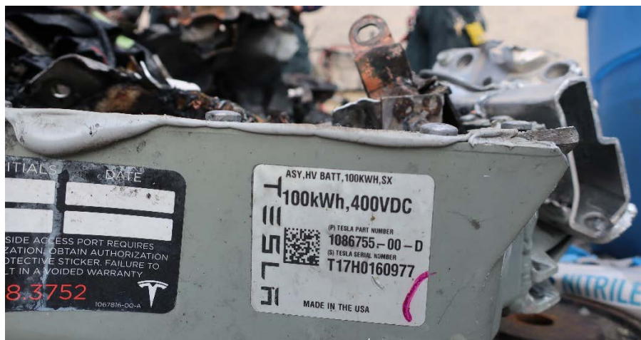
Figure 13. Battery identification sticker.
