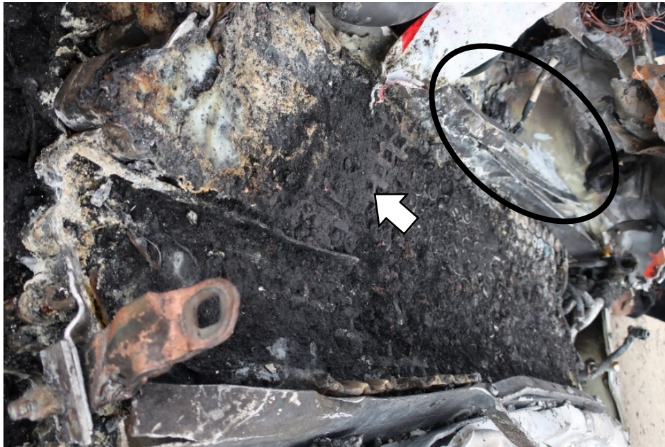
Figure 19. Top of module 15 after cleaning off debris from the fire. The forward edge is along the bottom of the photo. The arrow points to the edge of the top plastic tray. The oval indicates the partially open cover at the front of module 14. At the lower left is the module 15/16 bus bar.
