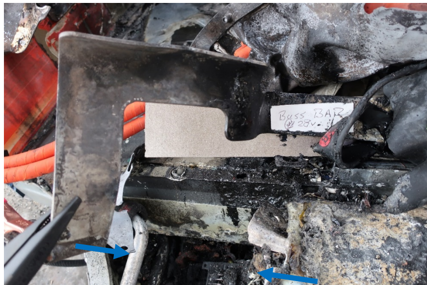
Figure 18. This captioned tag is on the 14 positive bus bar. The added blue arrows point to a fluid level, typical of burning above a fluid depth.
