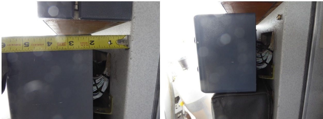
Photograph 2- FAP pulled away from the bulkhead.
