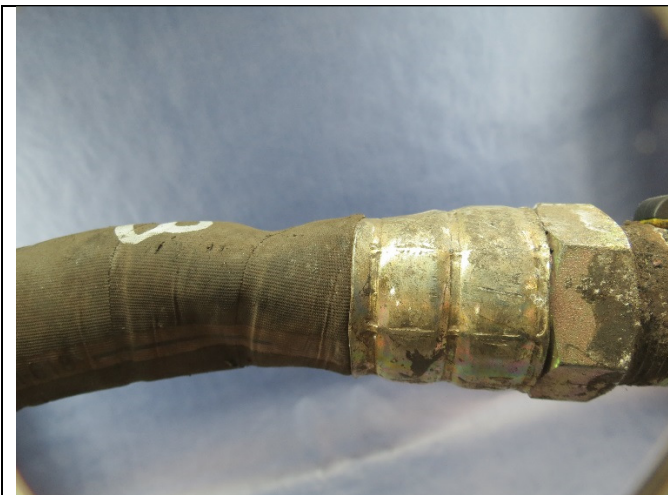
Figure 9A: Damage at end marked B3
