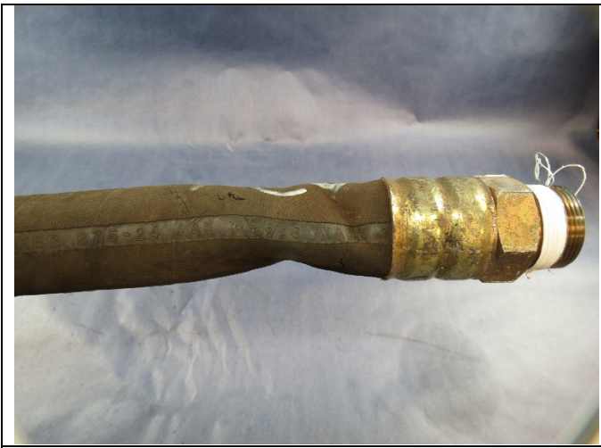
Figure 8A: Hose kinked at end marked A2
