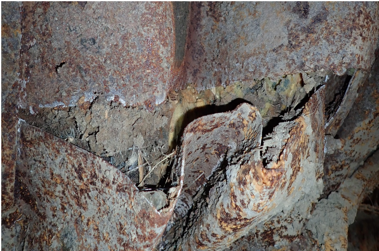
Vehicle Photograph: 6 - 2001 Ford Excursion Limousine – Image shows an opening in the floorboard due to corrosion. Interior carpet can be seen through the hole.
