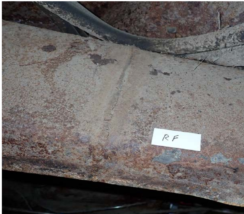
Figure 6: Right Front Frame Weld
