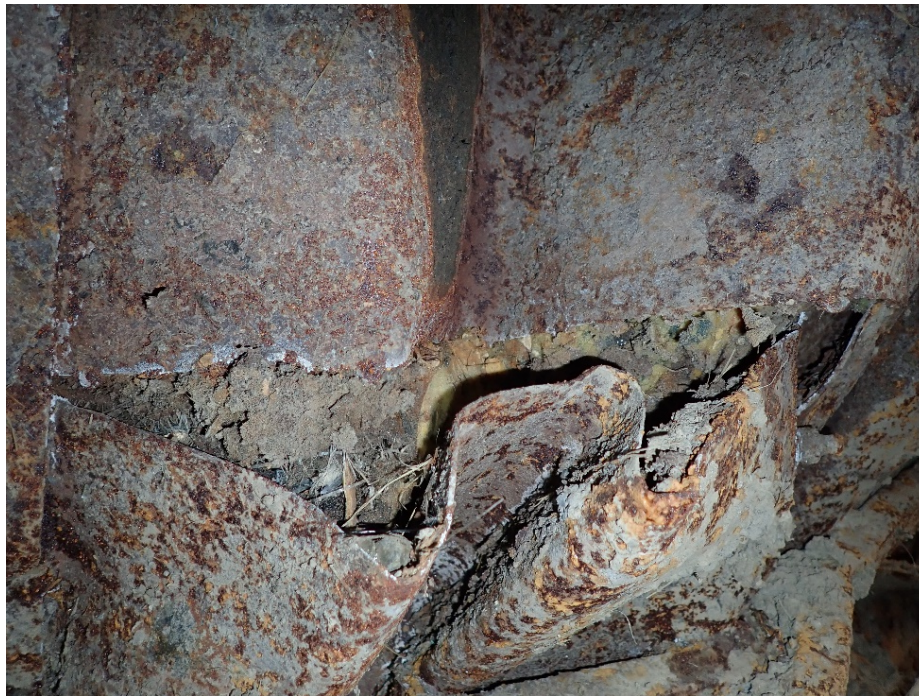
Figure 7: Opening in Floorboard
