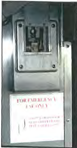
Figure 8: Emergency door release, FCA photo
