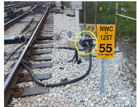
Figure 2: Signal Bond (circled), Wayside Track Circuit Sign and Cab Signal Sign
