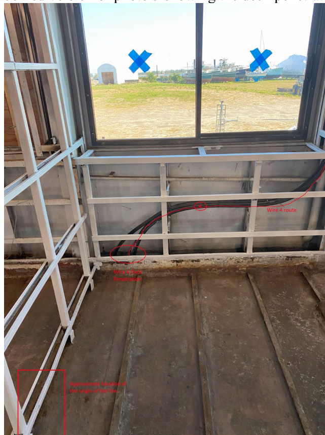
Photo 5- Showing the route of Wire 4 and the origin of the fire. Port side Outboard between FR57-60
