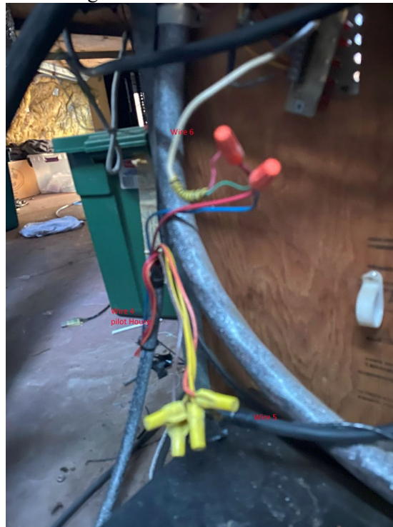
Photo 7- Showing Wire 4 where it terminates under the console in The pilothouse.
