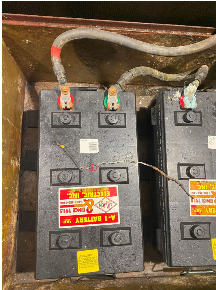
Photo 2- Port Main Engine starting batteries and the remains of Wire 1 Located just off centerline port between BH66 and FR64
