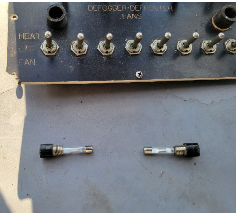
Photo 10 Wiper Panel with Fuses
