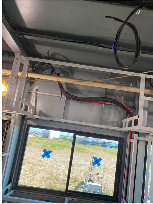
Photo 6- Showing the route of Wire 4 in the overhead of the main deck Connecting to Photo 5.
