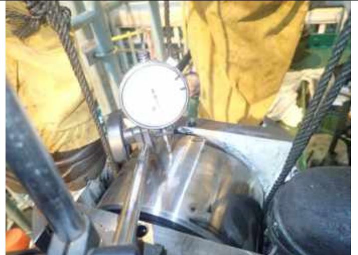
Measured clearance of roller guide
