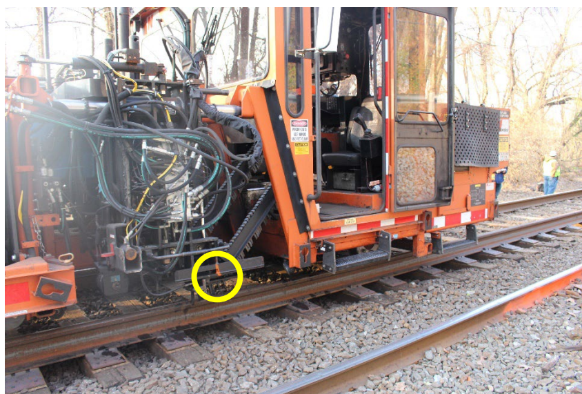
Figure 4 A photograph taken from the left side of the equipment showing distance traveled by the worker underneath the equipment and his final rest location circled in yellow. (Source: NTSB)
