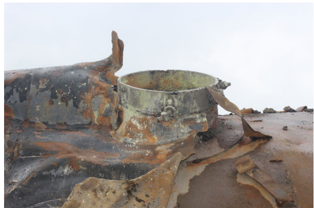
8(d) Manway cover missing.
