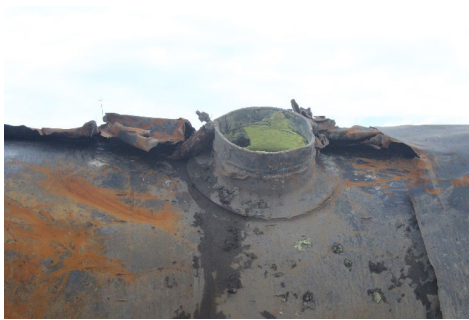
9(c) Manway with missing cover
