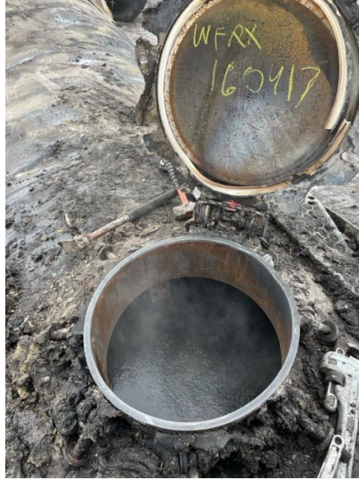
3(e) Showing thermal damage to manway gasket.
