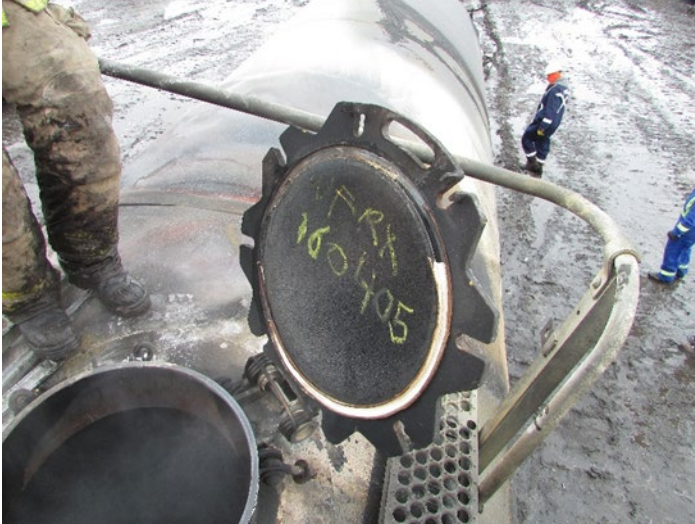
5(e) Thermal damage to manway gasket.
