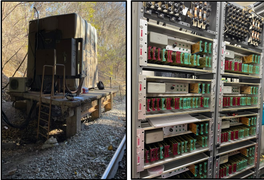
Figure 2: Signal bungalow on left and equipment rack on right.
