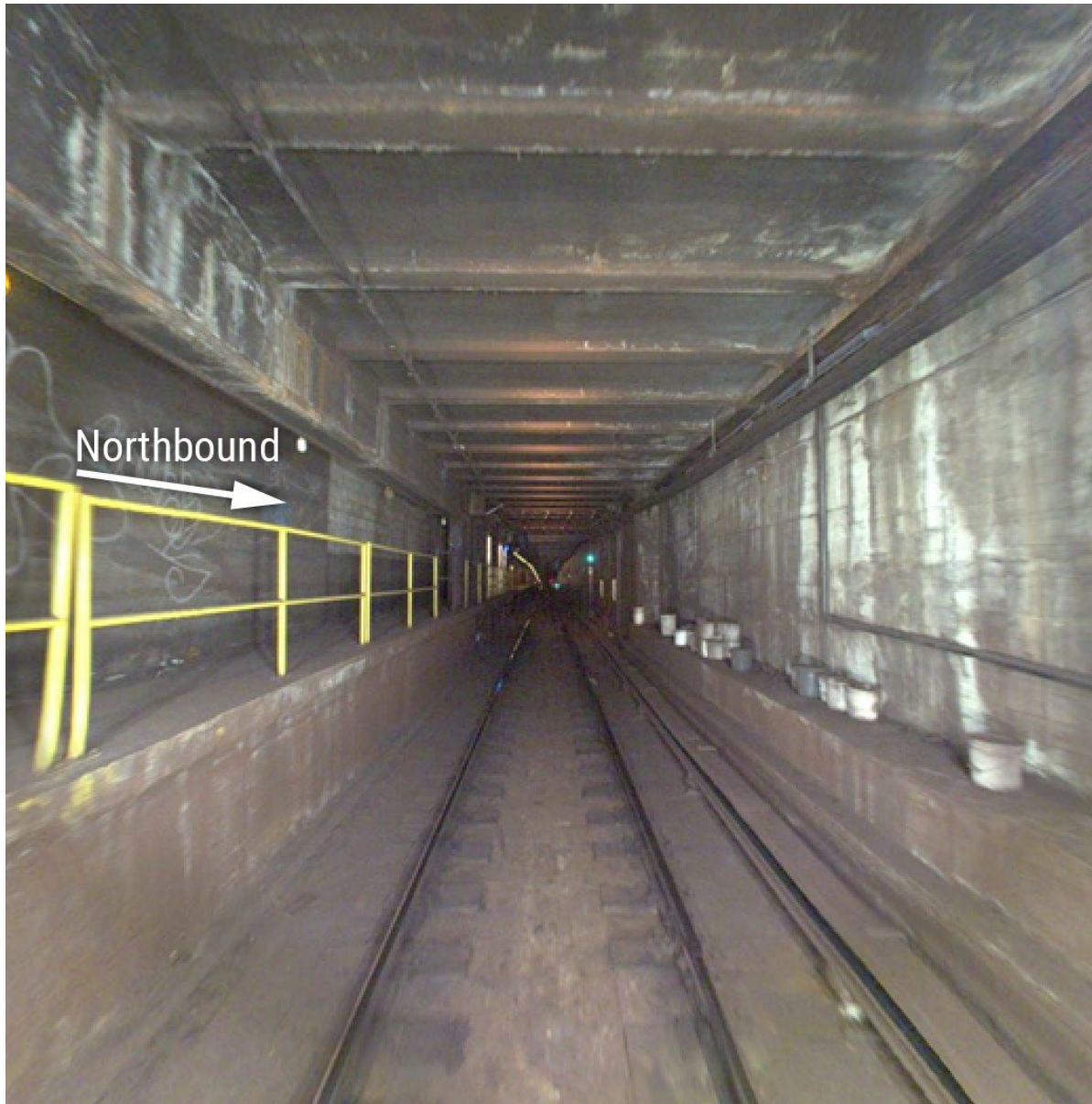
Figure 1 Photograph of accident seen looking north. Source NTSB
