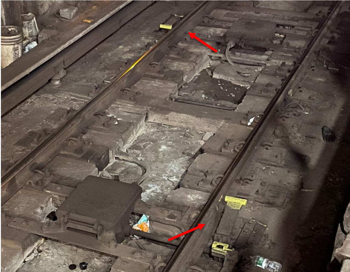
Picture 2: In-track automatic trip/stop system tied into the signal system.
