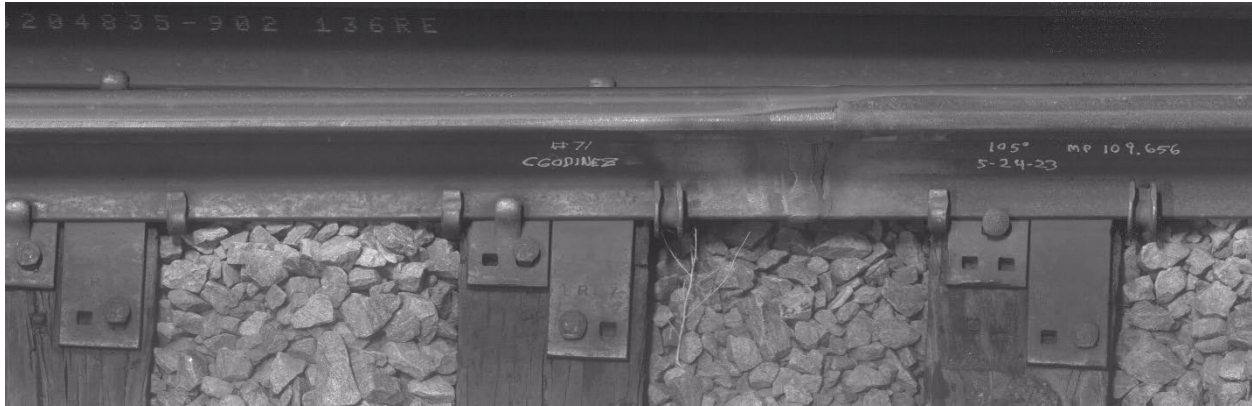
Figure 6. Image of thermite weld #71 on June 9th, 2023 (Source: BNSF)
