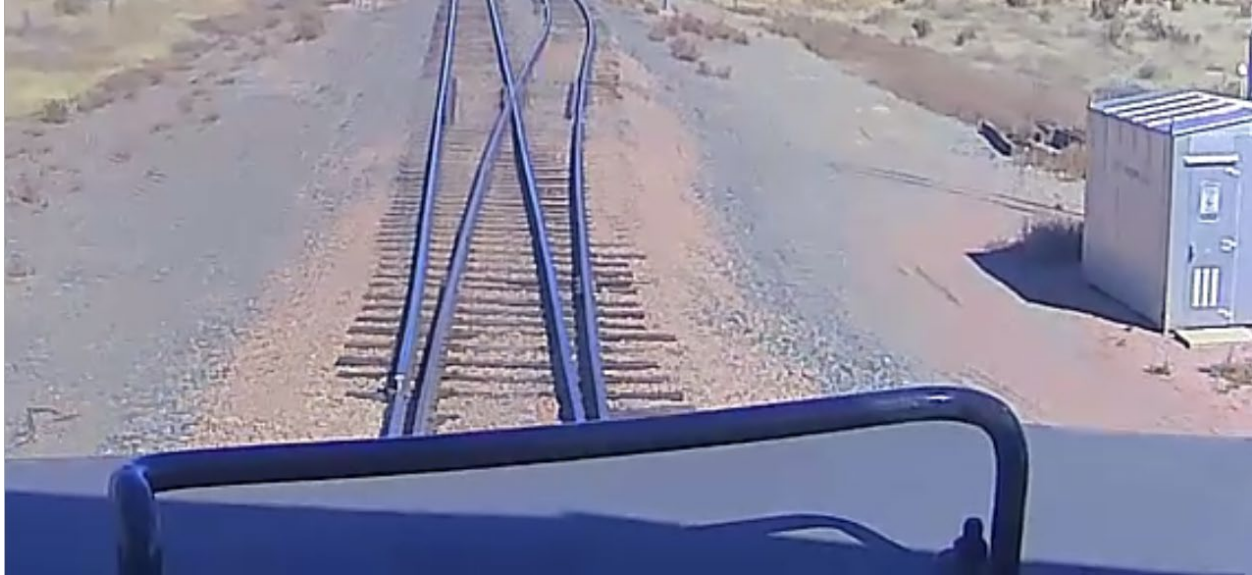
Figure 5. Still photo captured from the rear locomotive on BNSF train C-BTMSP50-33D, at 1:30 p.m. on 10-15-2023. The image shows a broken rail on the left stock rail that was not present on head-end video footage (Source: BNSF)
