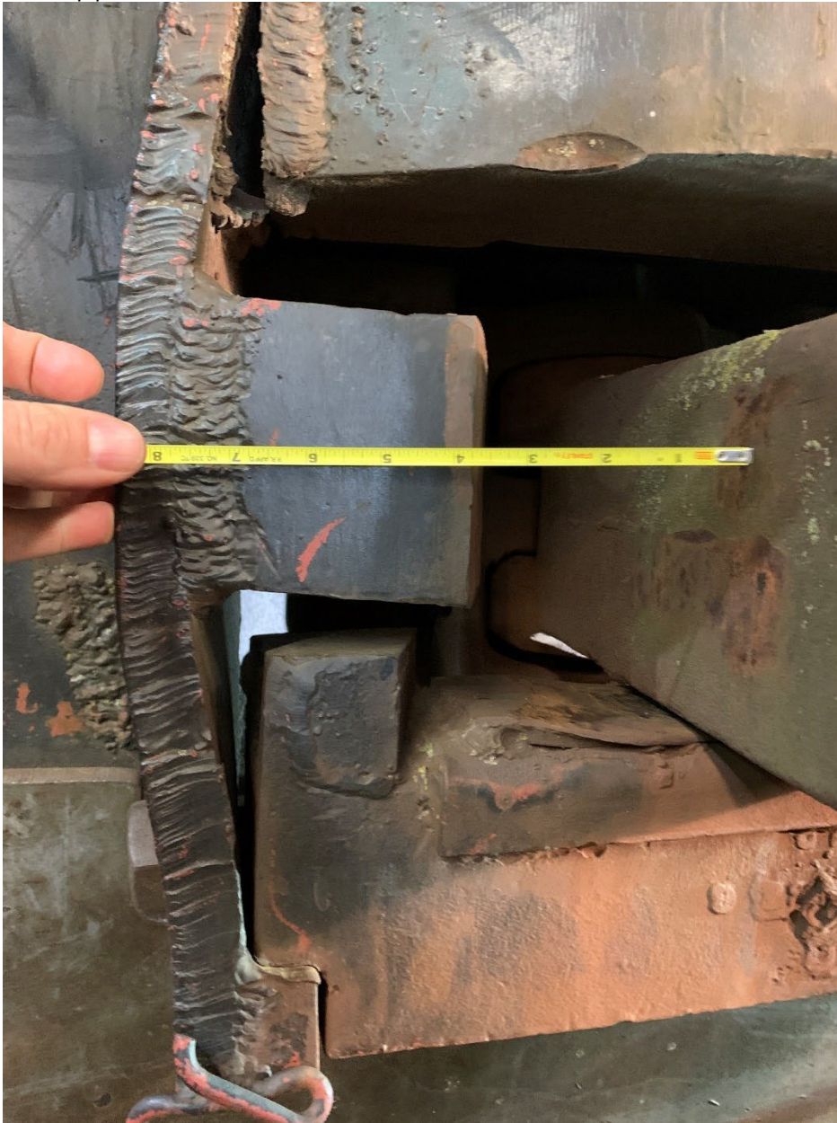
Figure 19. Draft gear pocket of RME8 08, left rear location
