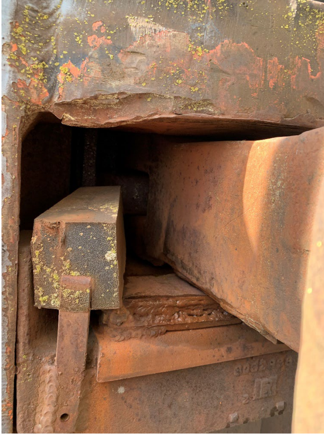
Figure 20. RMEX 06 Pennsy coupler alignment block, improperly secured with weld.
