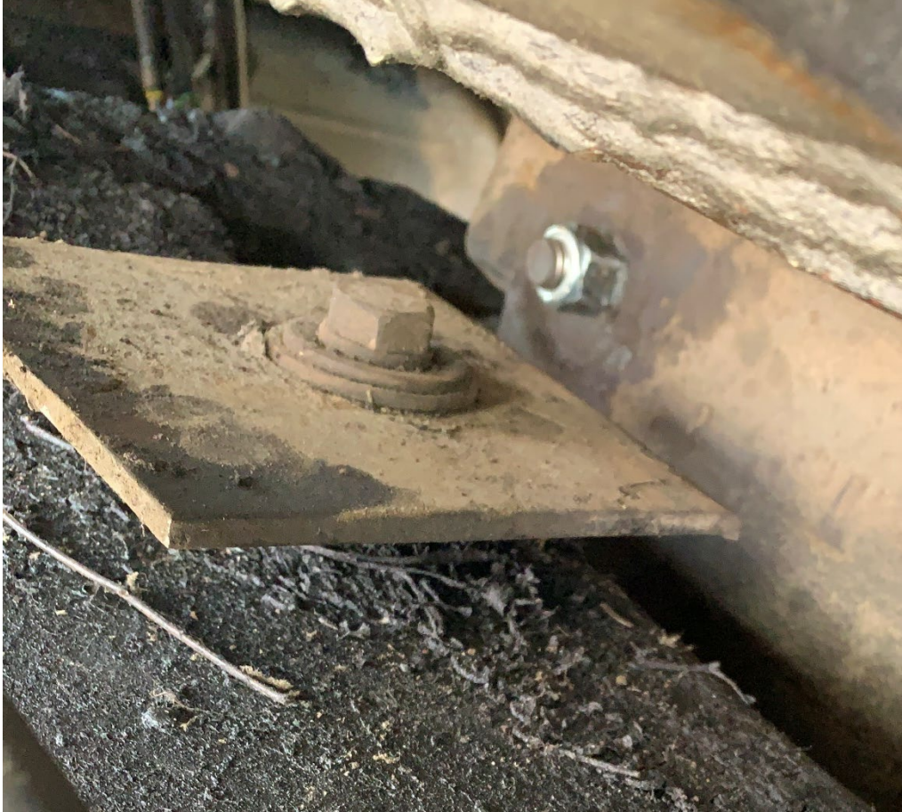
Figure 41. RMEX 08 broken bolster stop block
