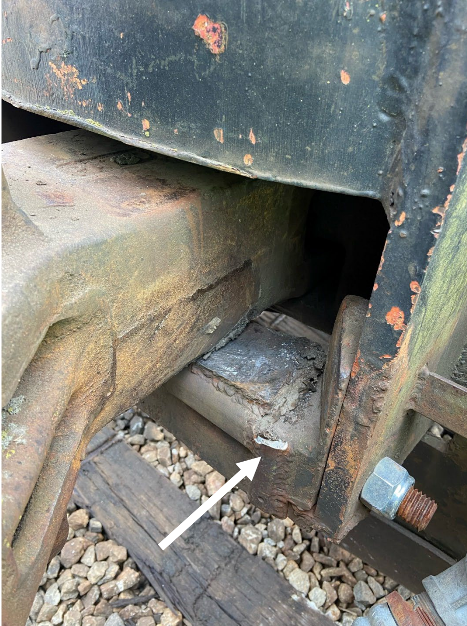
Figure 22. Draft gear pocket of RMEX 06 left rear location, showing broken coupler stop bracket.
