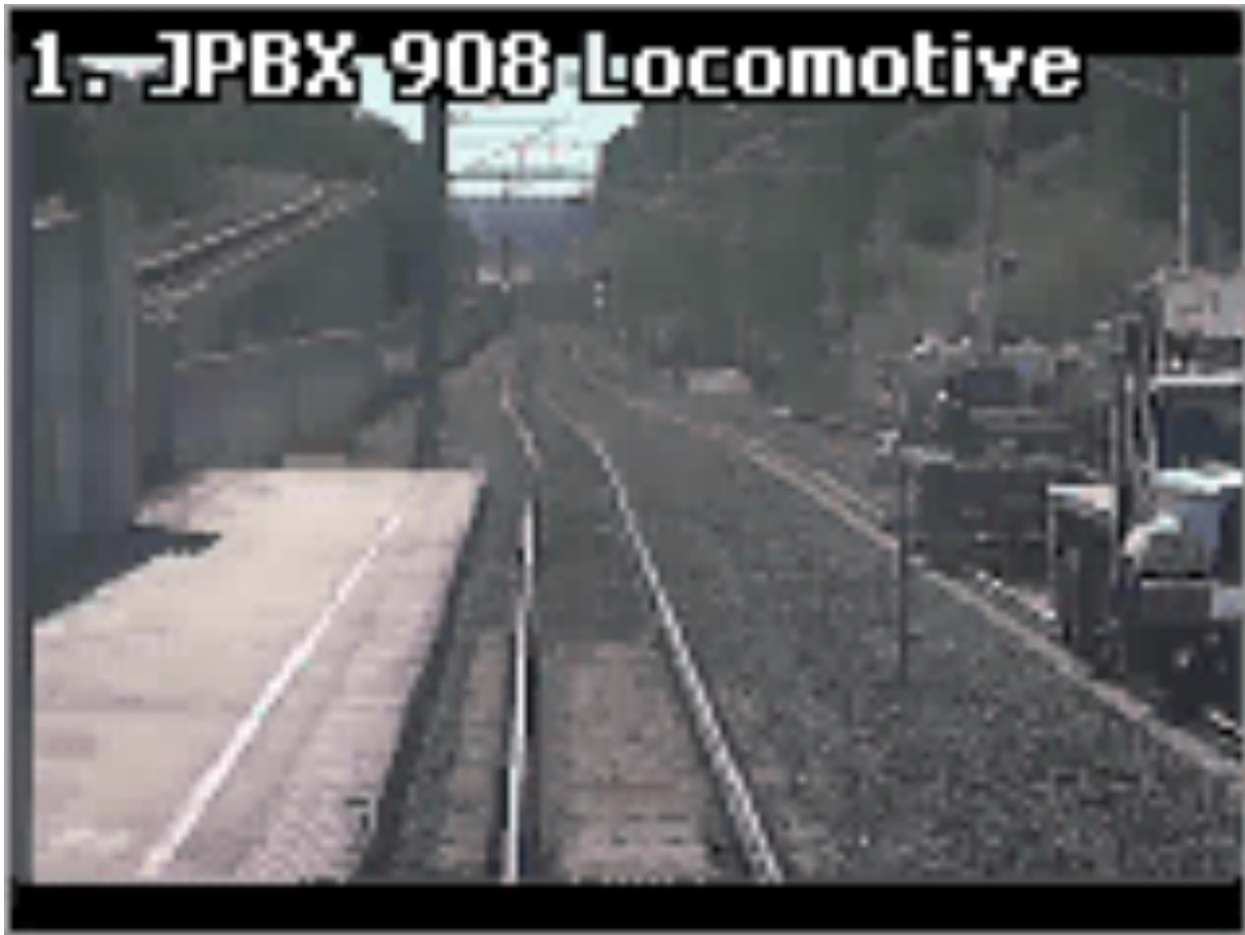
Figure 3. View of the rear of the work convoy on the parallel track.
