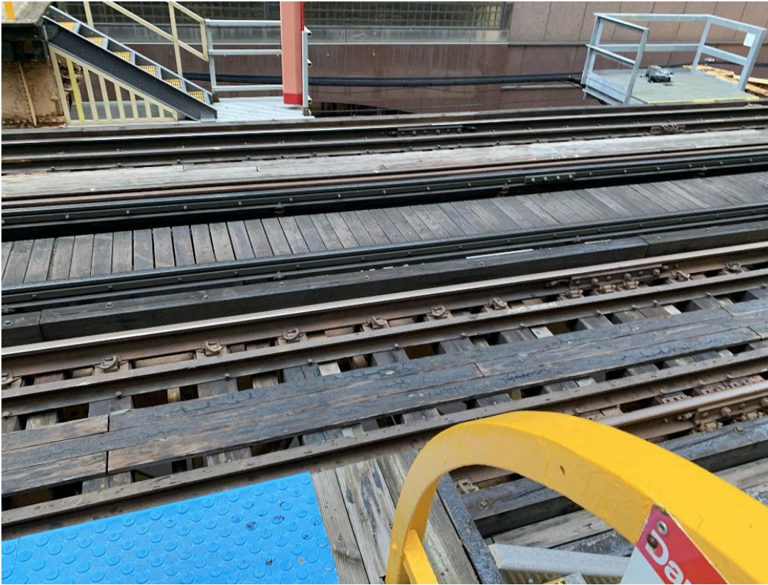
Figure 7: Photo shows the area of the accident.
