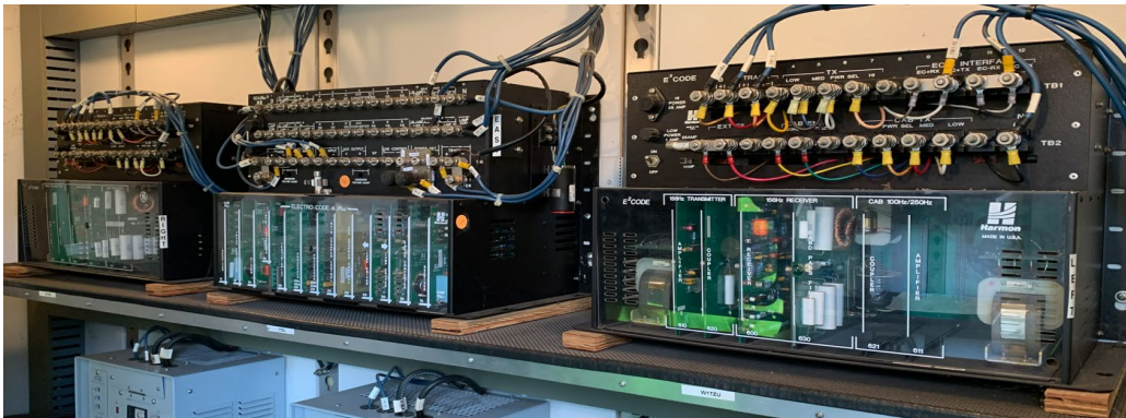
Photo shows the multiple Electro Code units used to detect track occupancy for the signal system
