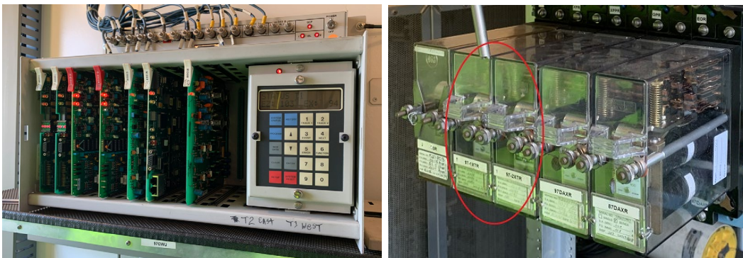
Photo to the left shows Safetran 3000 unit. Photo to the right shows the 2 D.C. track relays
