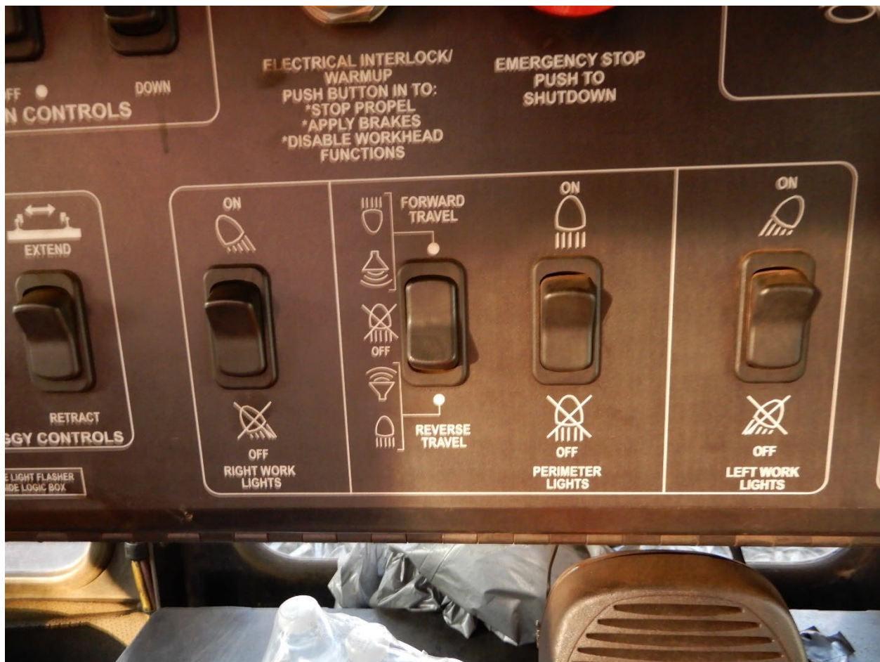
Figure 6. GS 15022 MCC with Forward/Reverse Travel Switch located in the center of the photograph. Icons indicate the intended function of lights/alarms. (NTSB Photograph)
