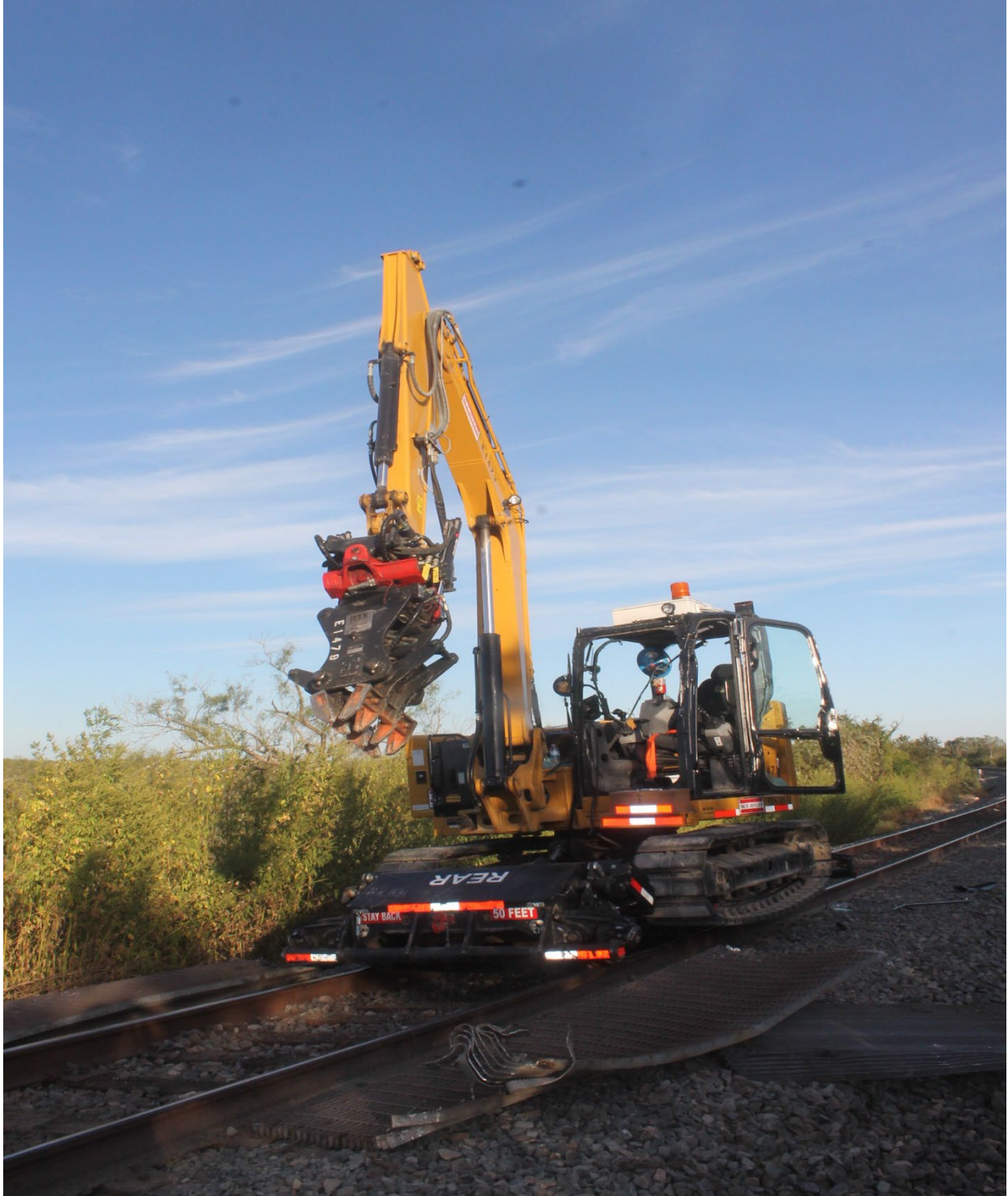
Figure 2- photo of the accident equipment at the accident site
