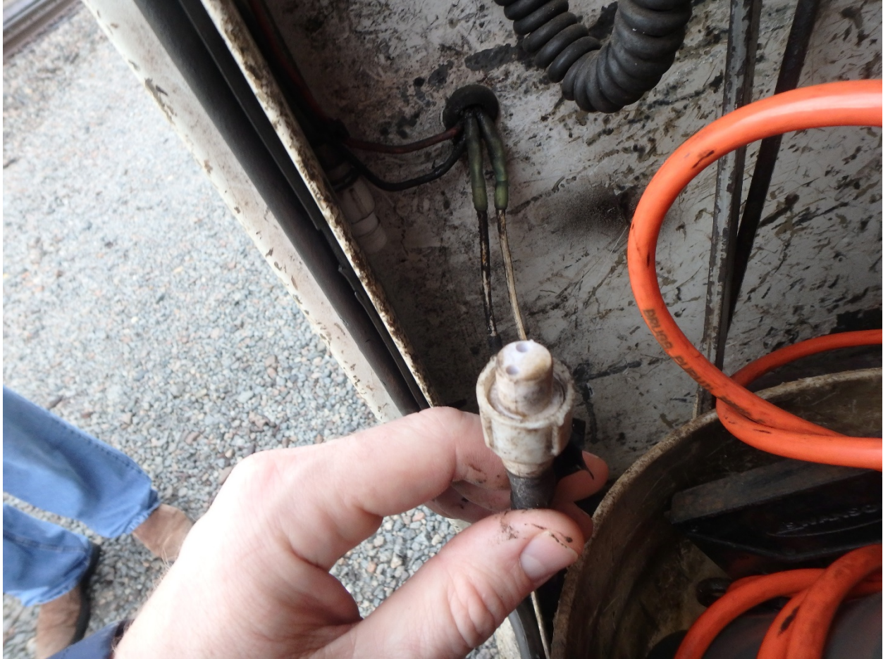
Figure 5. Photo showing disconnected wire connector that was intended to connect the external mounted speaker to the external radio. The wire was disconnected from the radio and hanging inside the cabinet.
