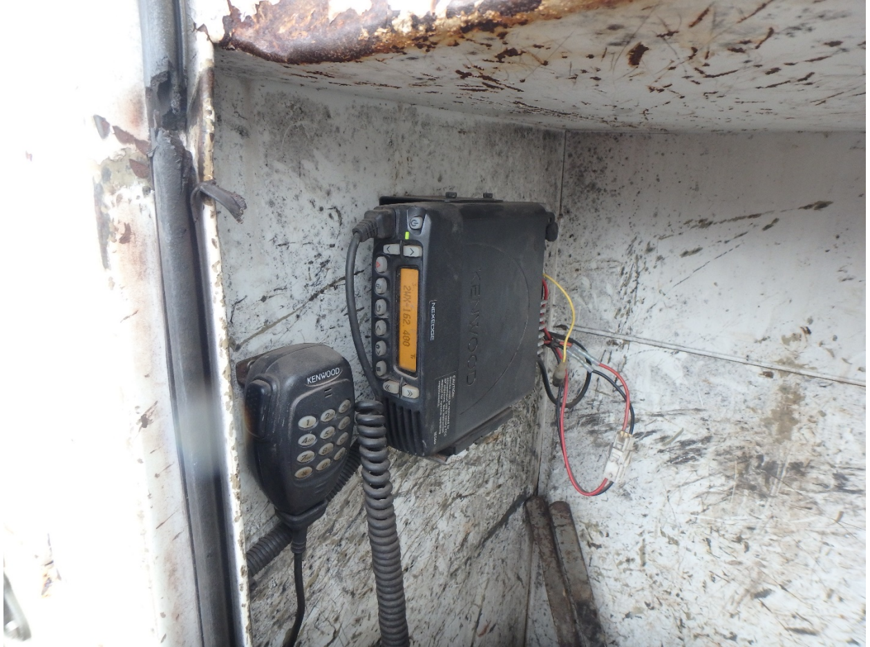
Figure 4. Photo showing the external radio mounted inside of a cabinet on the body of CSX welding truck No. 240150.
