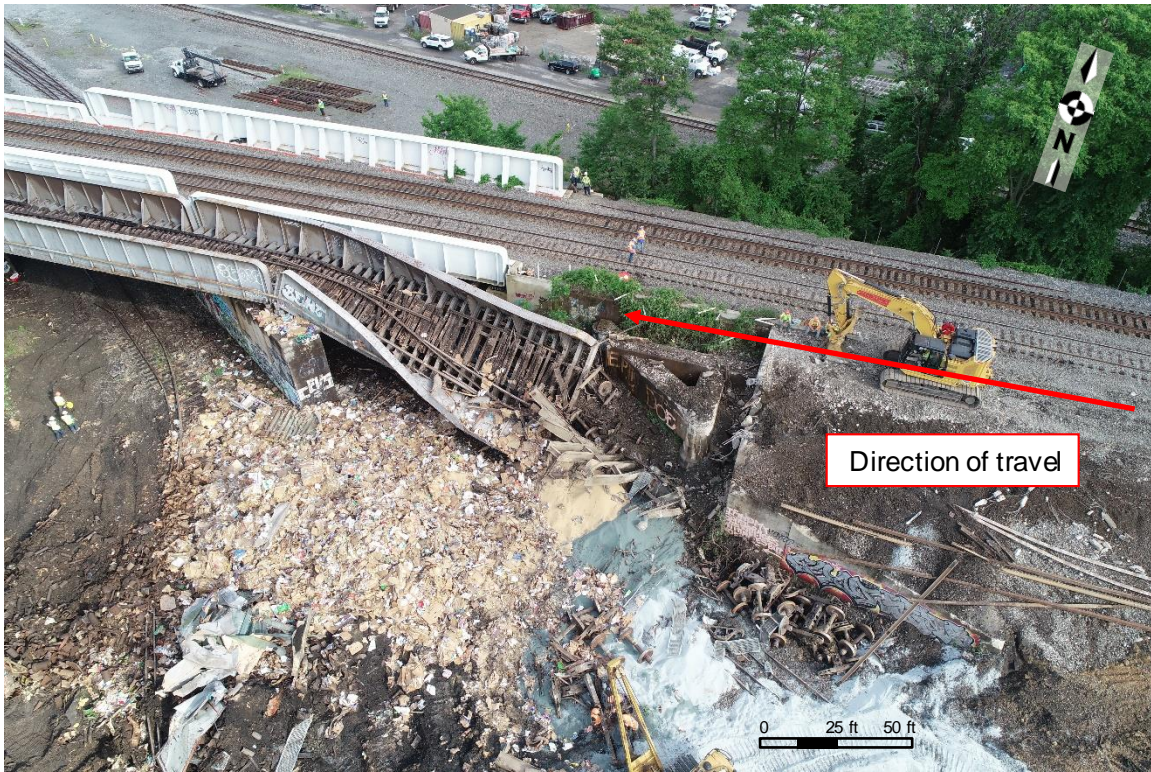
Figure 1 – Photo of collapsed bridge area
