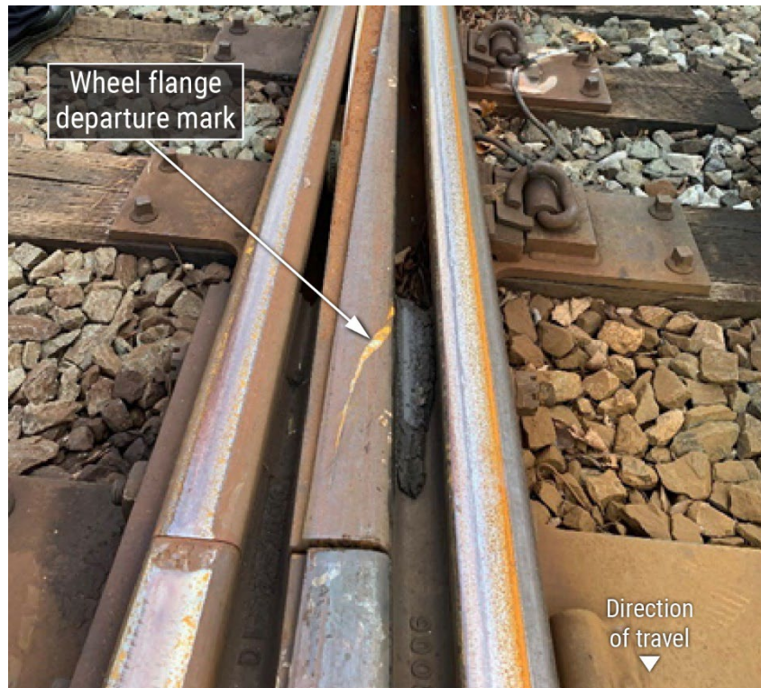
Figure 5. Wheel flange departure mark on the switch point guard near the heel of 1A switch.
