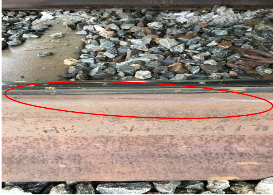
Figure 3. High rail with the flange mark circled in red.
