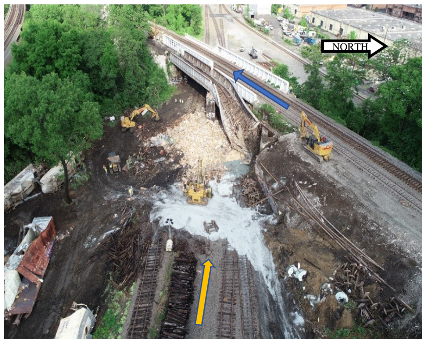
Figure 1. The damaged bridge. The blue arrow indicates the direction of travel on the CSX track and the yellow arrow indicates the NS tracks.
