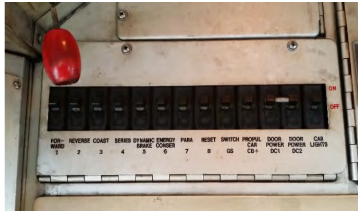
Inside #1 Cab Above the high voltage circuit breakers (Above Cab Seat)
