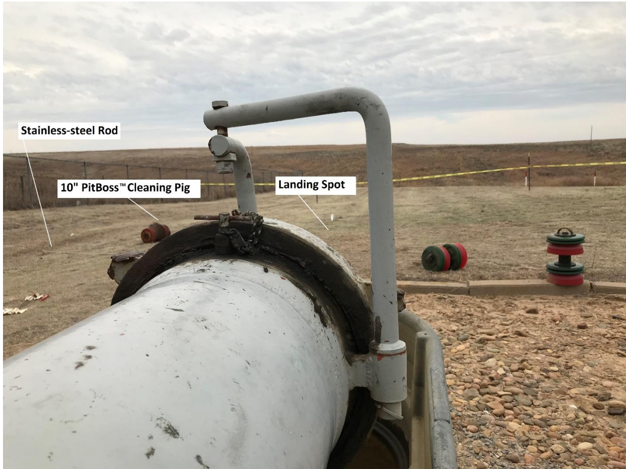
Figure 6. Photograph of End of East 10" Receiver Facing South Please Note the Flag where Technician 1 Landed and the Position of the 10-inch PitBoss™ Cleaning Pig Rodriguez, March 28, 2020
