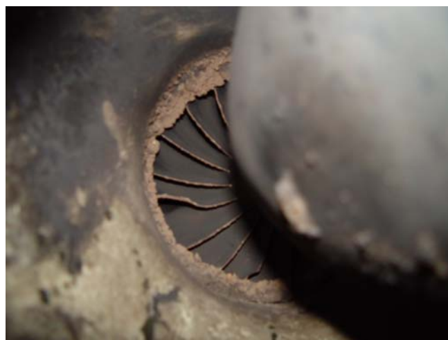
PHOTO 2: LT ENG 1 ST -STAGE IMPELLER DAMAGE
