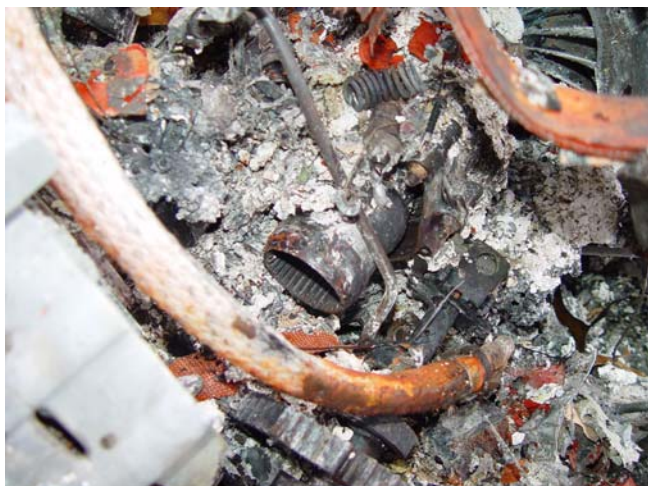
PHOTO 4: ACCESSORY GEARBOX DAMAGE
