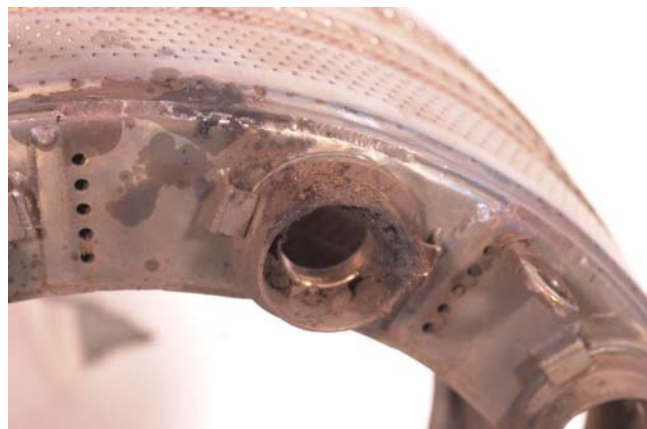
PHOTO 10: DEBRIS IN COMBUSTION CHAMBER
