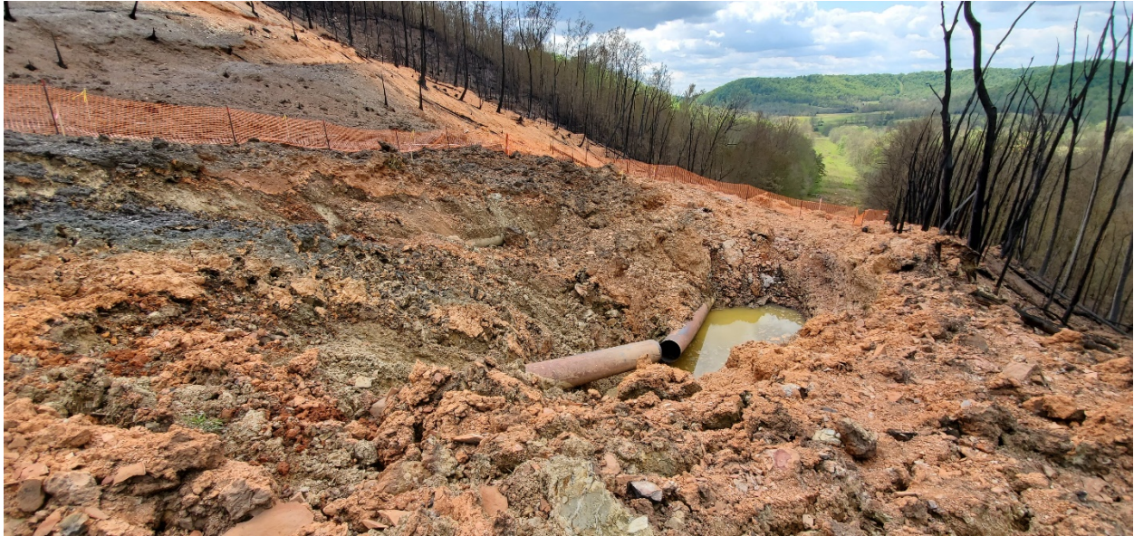
Figure 10. Site surrounding ruptured girth weld, taken May 7, 2020 at 1:42PM (Courtesy of BGC)
