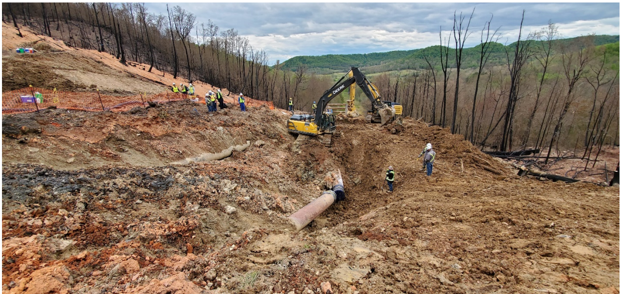
Figure 11. Site surrounding ruptured girth weld during excavation, taken May 11, 2020 at 4:57PM (Courtesy of BGC)
