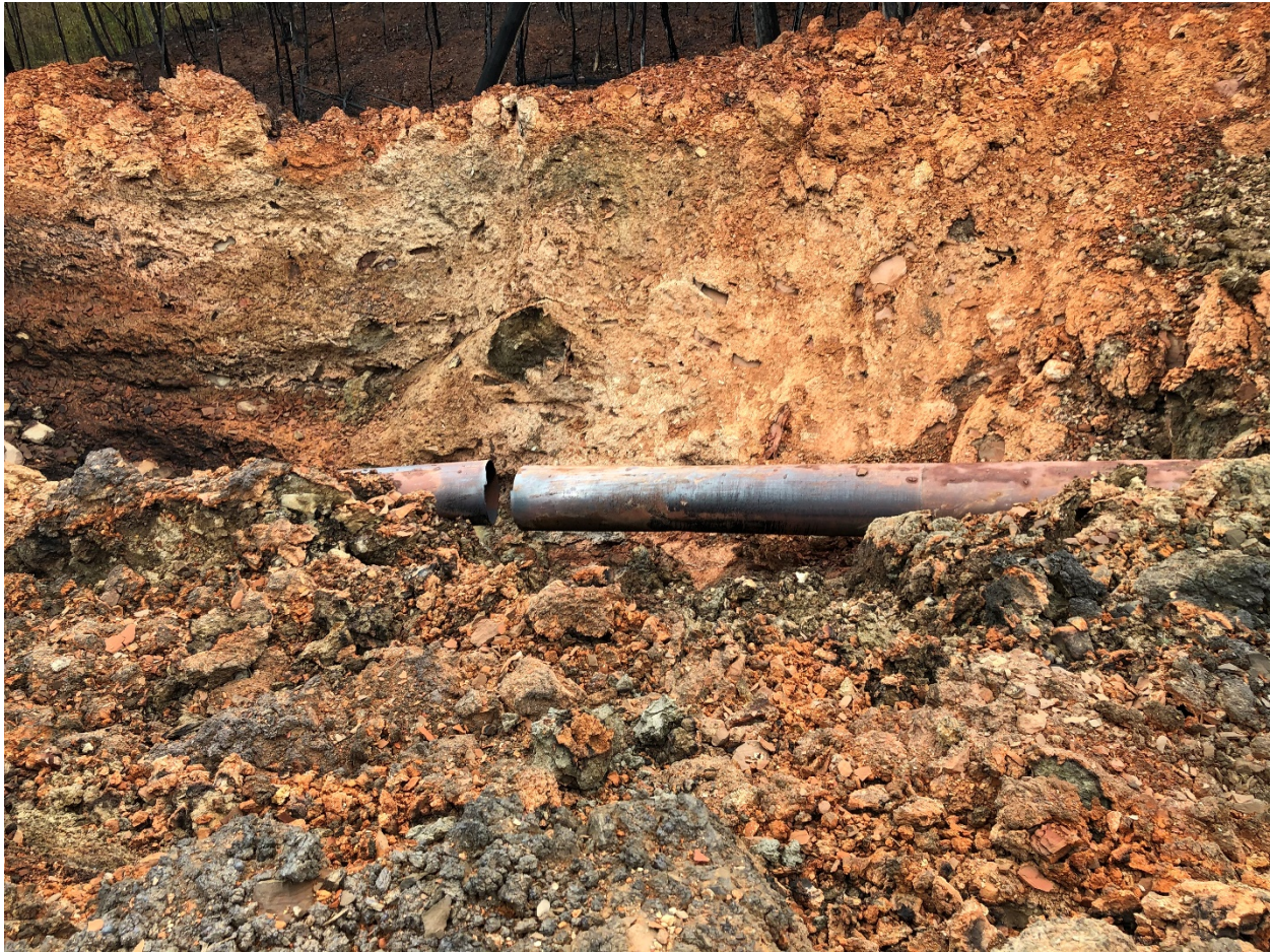
Figure 8. Ruptured girth weld, taken May 5, 2020 at 12:11PM (Courtesy of Enbridge)
