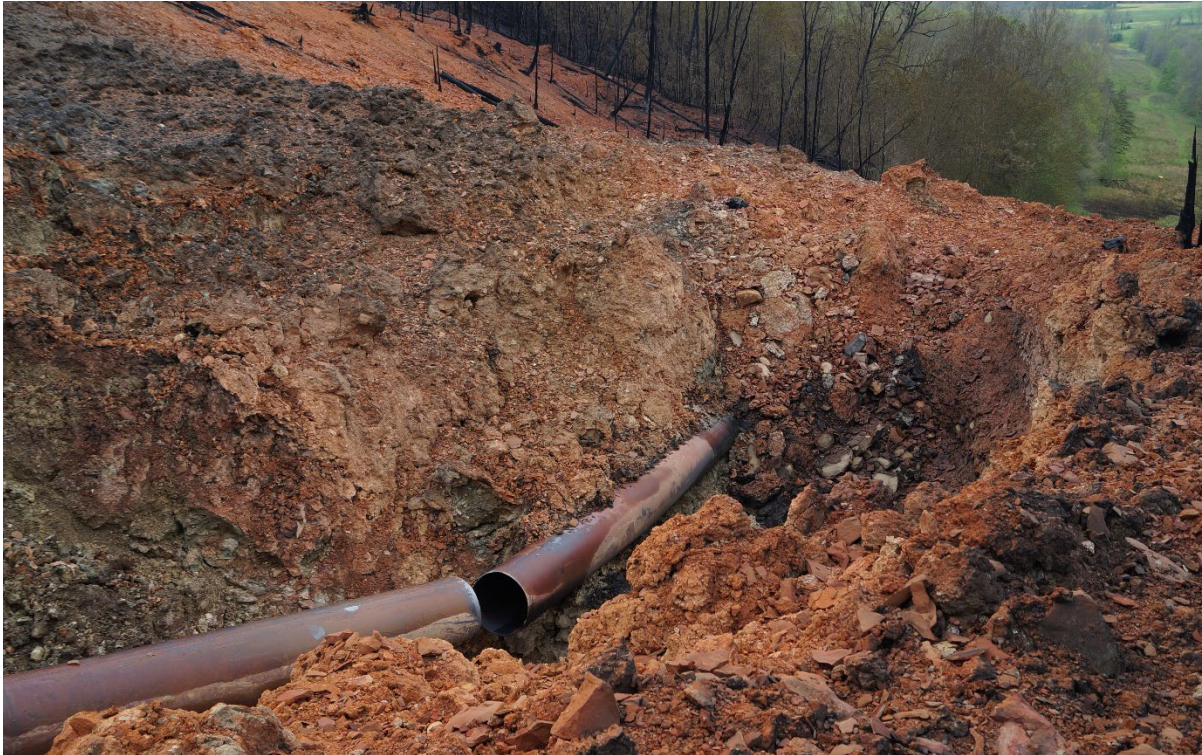
Figure 4. Accident Site Post-Rupture, Taken 5/5/2020 (Courtesy of PHMSA)
