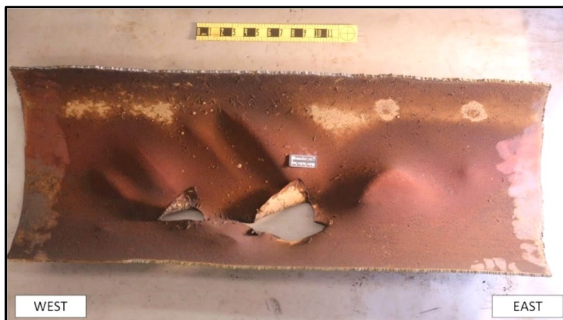
Figure 33. Interior surface of pipeline coupon encompassing all visible damage. NTSB preliminary examination photograph, December 10, 2020.
