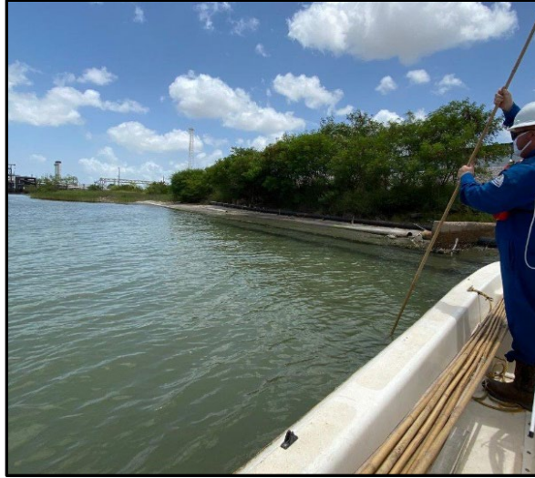
Figure 17. Enterprise pipeline technician setting cane poles to mark pipeline TX219 in the vicinity of the accident, July 16, 2020, courtesy, The Orion Group.
