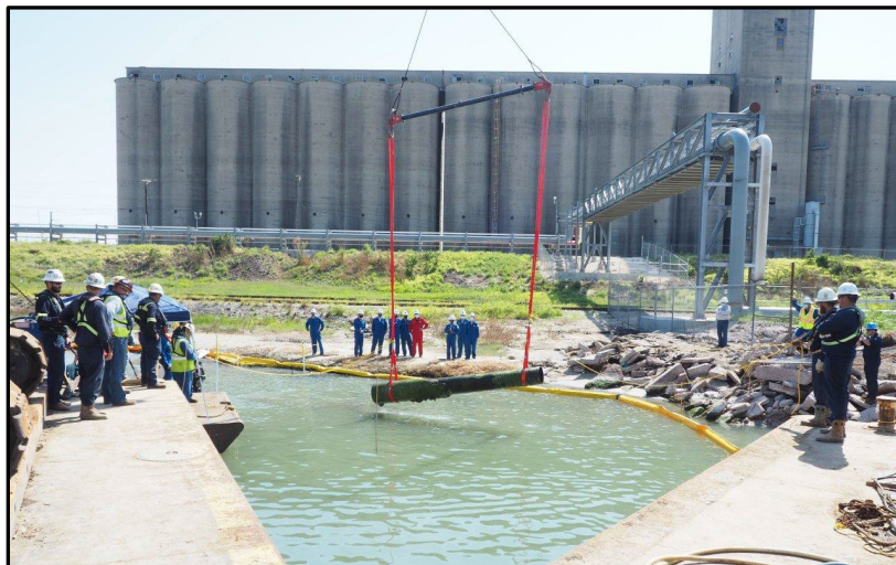
Figure 30. Photograph facing south toward the shoreline as Enterprise Products crews and contractors rigged the extracted damaged pipeline segment from the accident location, October 5, 2020. Courtesy, Enterprise Products.
