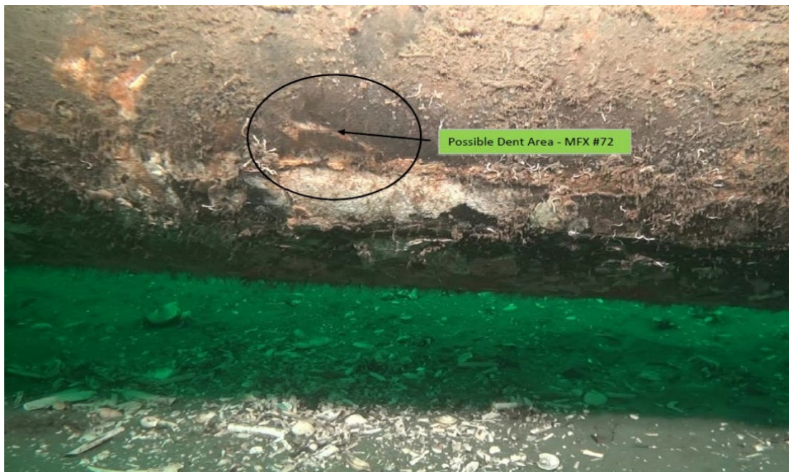
Figure 23. The October 2021 ROV survey showed a possible dent with missing coating. Photograph by Aqueos, October 15, 2021.
