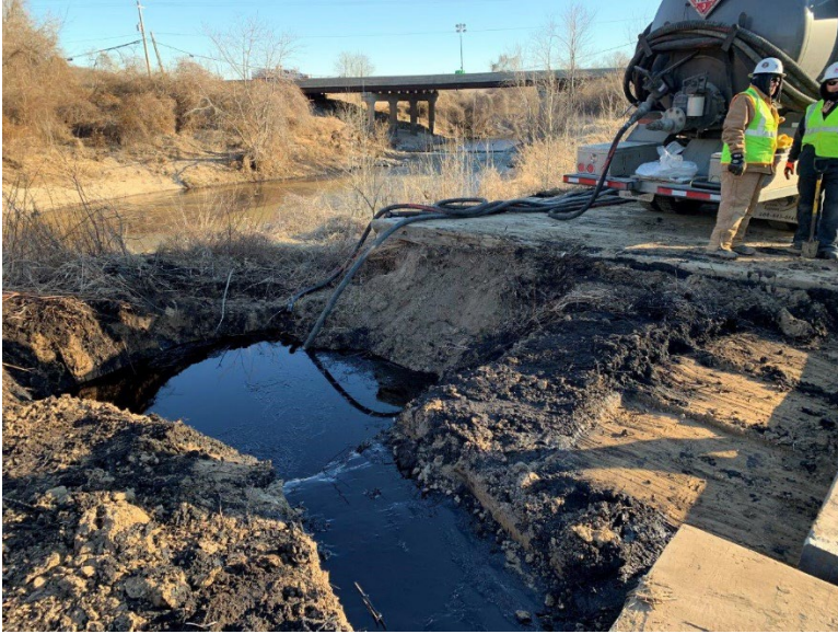
Figure 8. Diversion ditch and pothole at source area, March 12, 2022, 11:36.
