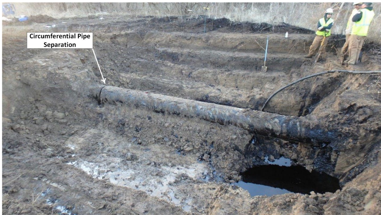
Figure 3. Excavated pipeline at the breach location and circumferential pipe separation, March 12, 2022, 17:27.
