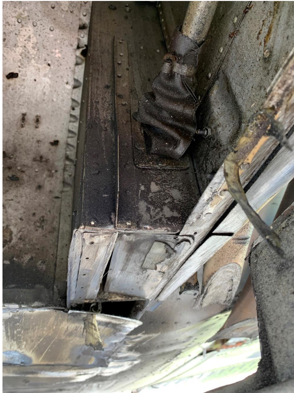
Photo 1 – Engine Keel Beam Damage (Courtesy of FAA)
