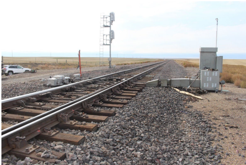
Figure 16 A photograph of the track switch heater in place at the Buelow West track. The switch heater sits 11 feet back from the track. The duct work and connecting hoses feeds propane from a tank (not pictured) to heat the track surface. (Source: NTSB)
