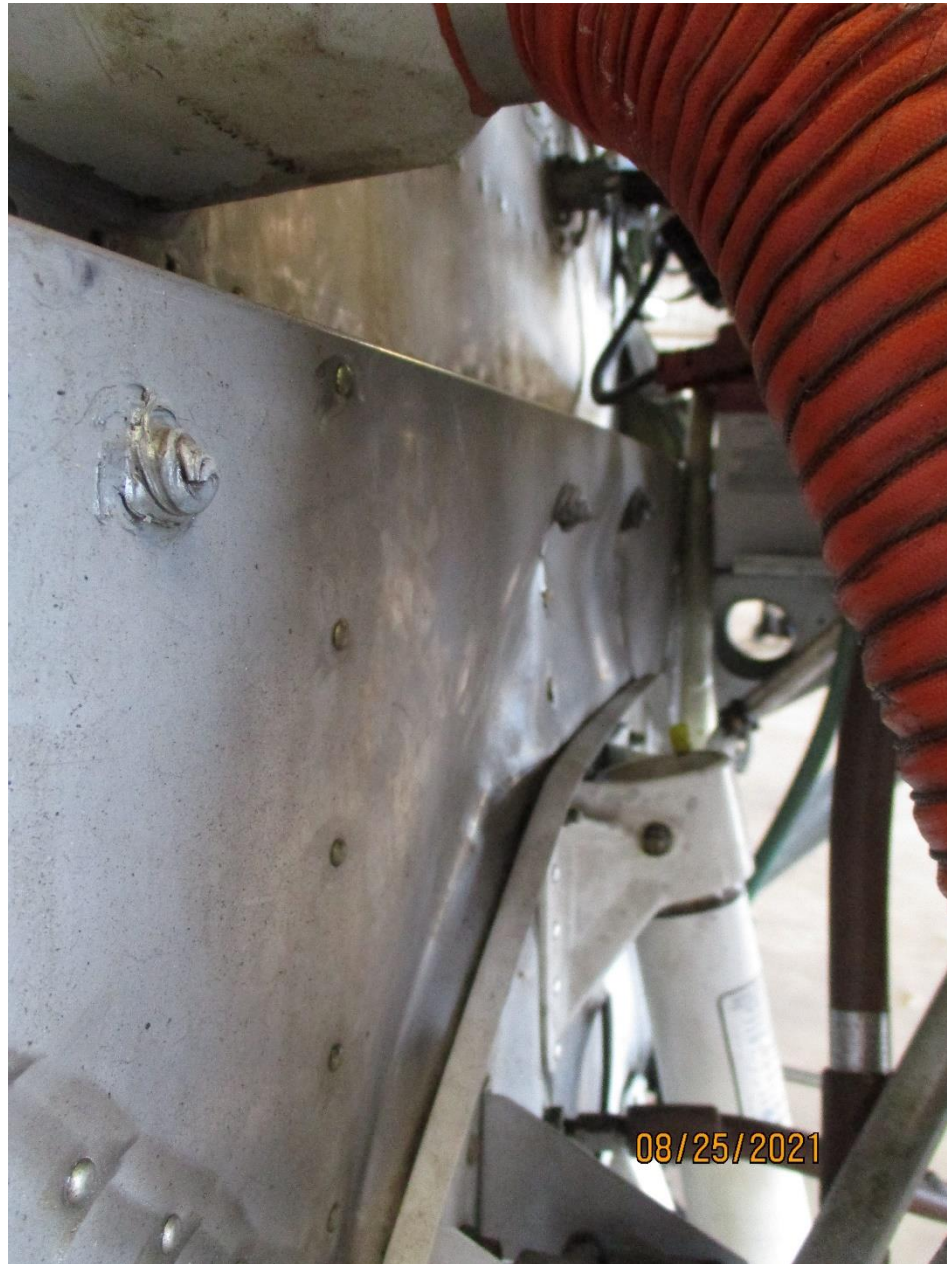
Photo 2 – Firewall Damage (FAA Photo)
