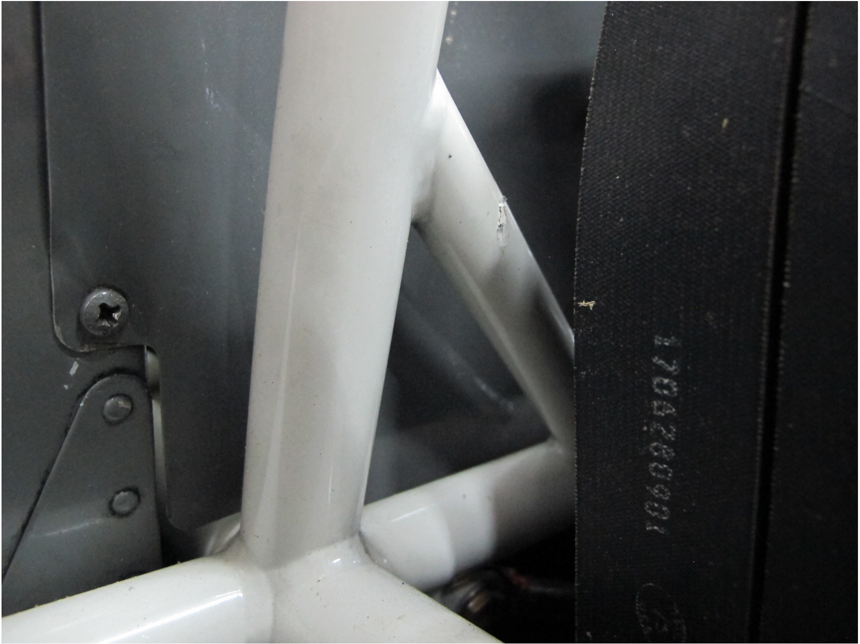
Photo 4 – Sheave Impact Mark
