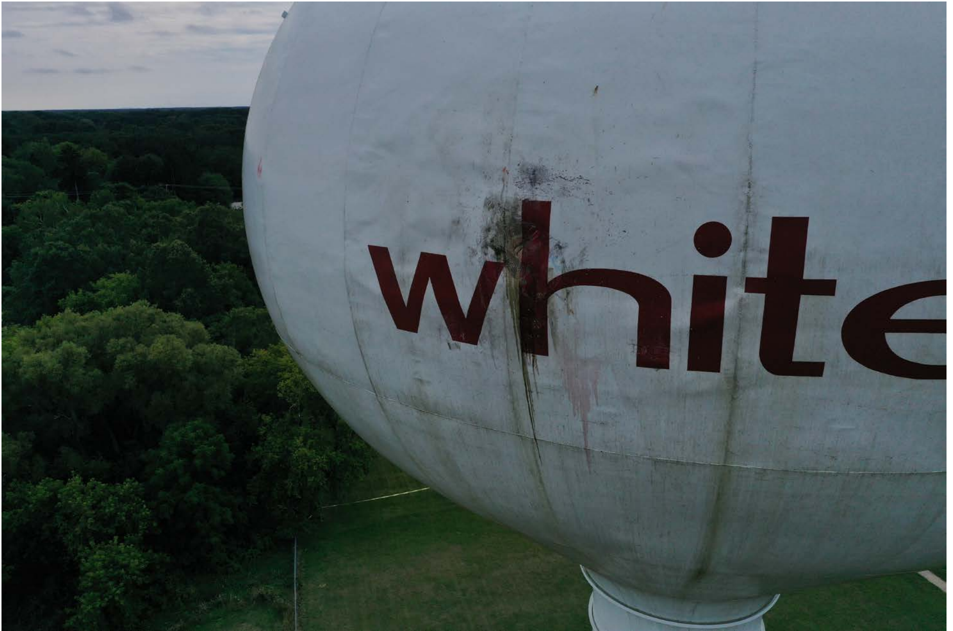
Photo 3 – Water Tower Damage (White Lake Fire Authority Photo)
