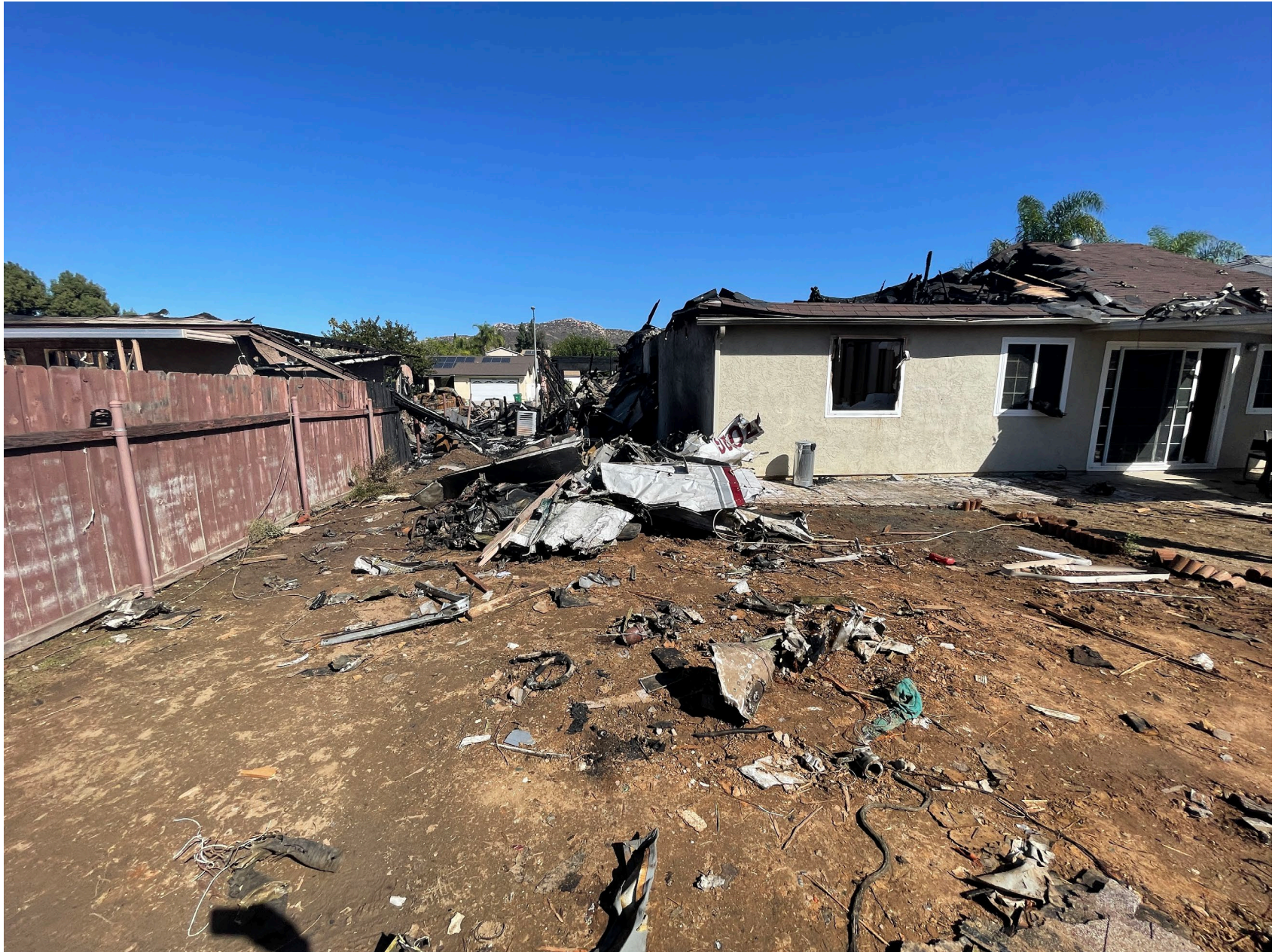
Photo 3 - View of the accident site.
