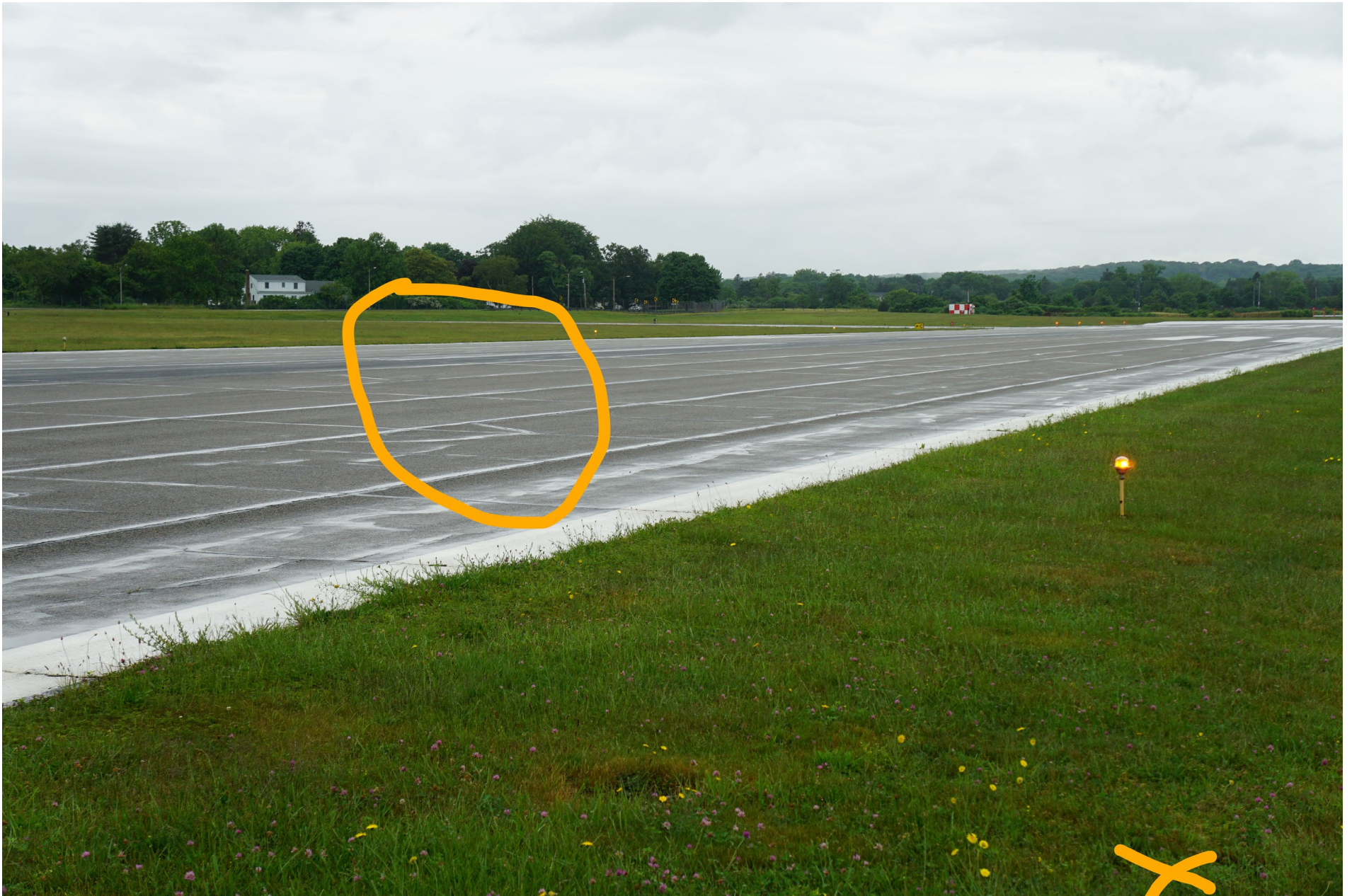
Photo 6 – Runway Tire Marks (FAA Photo)
