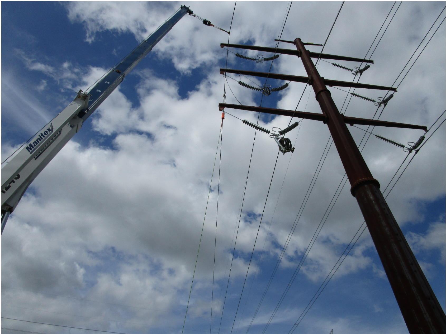
Photo 4 – View of power lines and the long line leading toward helicopter (Photo Courtesy of FAA)
