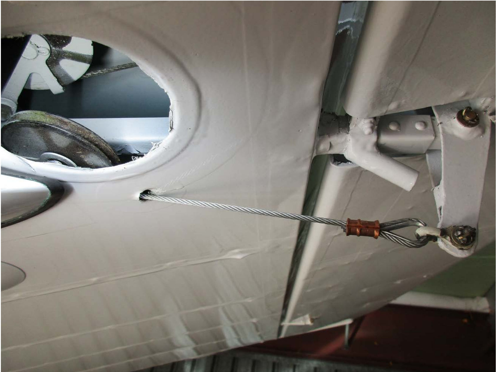
Photo 4 – View of the right aileron bellcrank. (Photo courtesy of the FAA)
