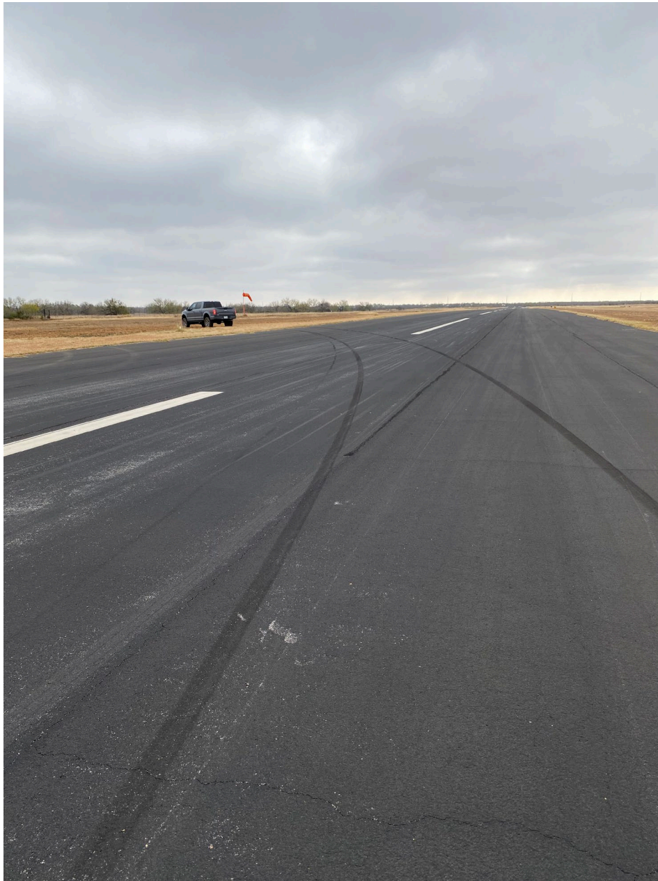
Photo 2 – Tire Skid Marks on Runway 13 (Source FAA)
