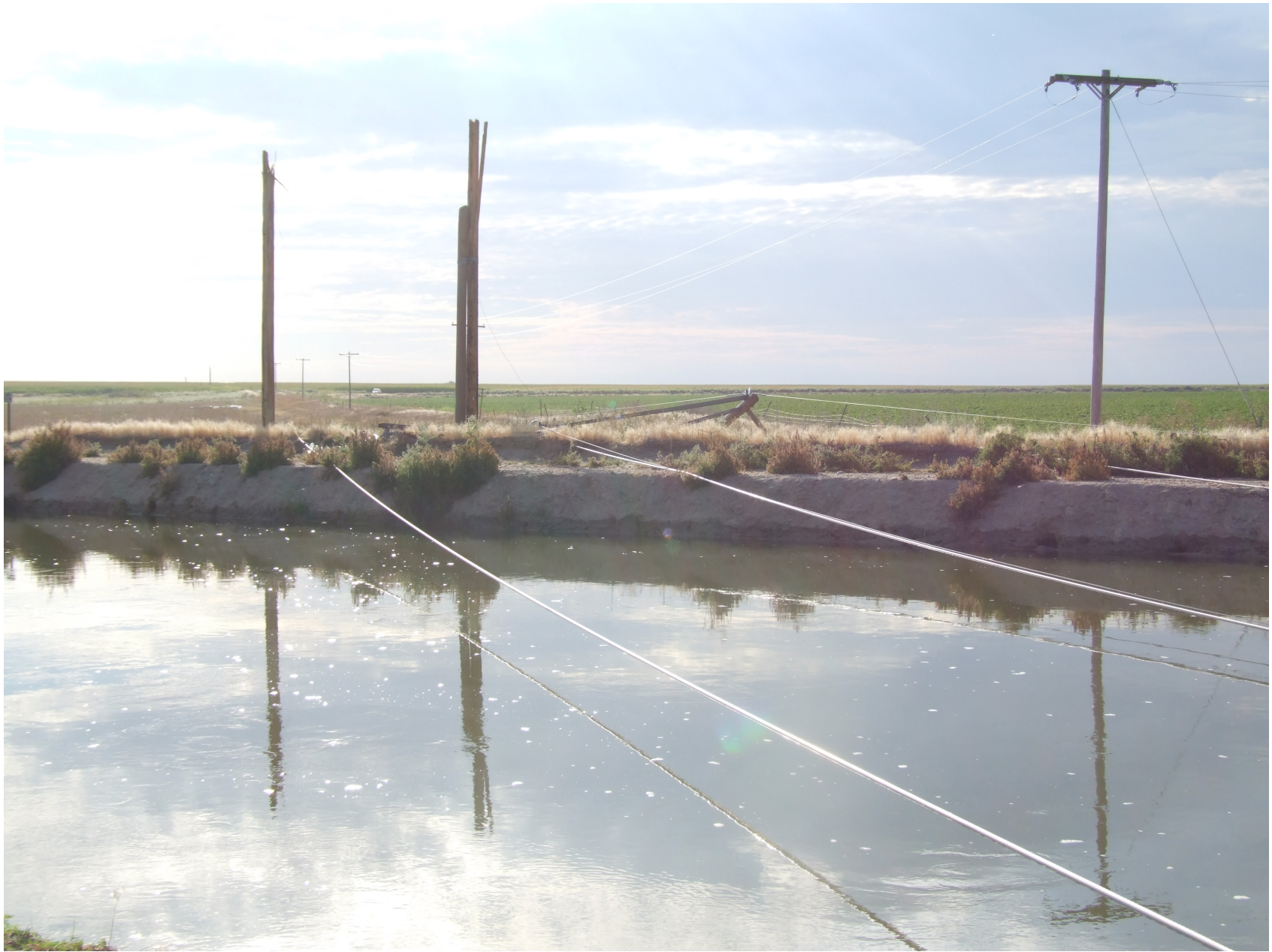
Photo 4 – Downed Power Lines
