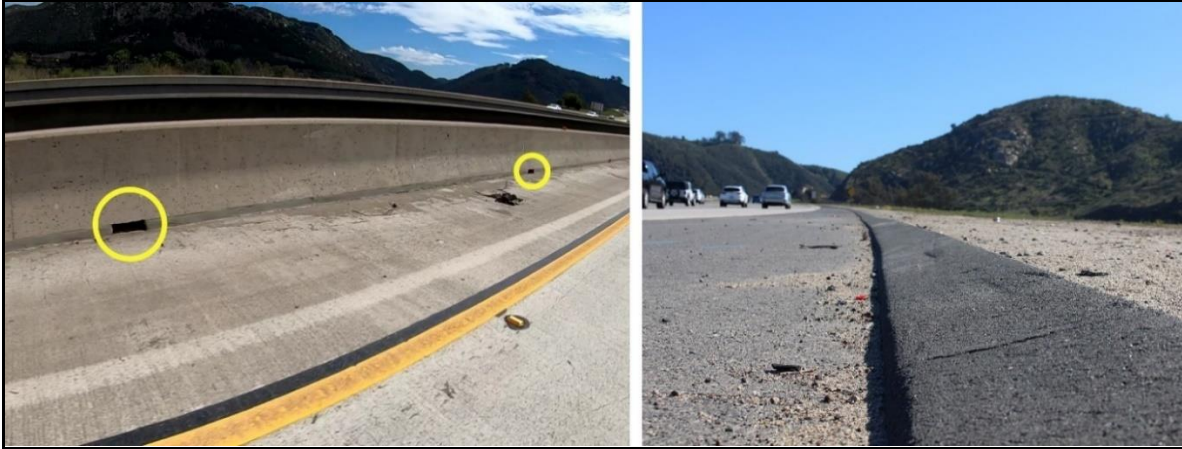
Figure 6. Drainage devices along southbound lanes in area of crash. Depicted are (left image) scupper drains along the left shoulder on the bridge and (right image) a drainage dike along the right shoulder past the bridge.
