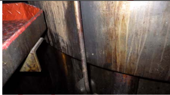
Return pipe for fuel valves incorrectly mounted, pipe hanger missing.
