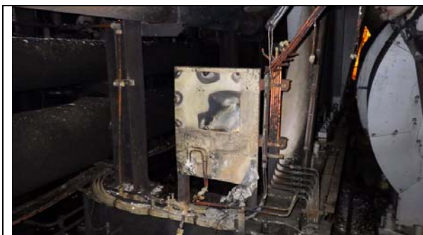
Entire control panel for turbo charger cut out missing (melted)
