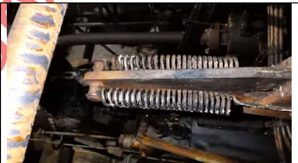
Fuel rack lever and springs exposed to extreme heat
