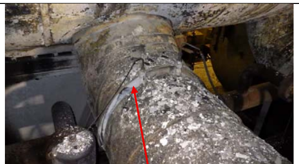
Exposed compensator flange where the fuel oil/gas oil caught fire.
