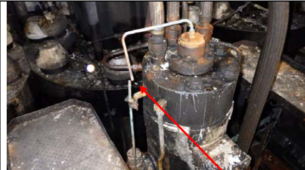
Fuel pump top cover with puncture valve. Brass fitting, straight male coupling, for puncture valve copper tube missing (melted)
