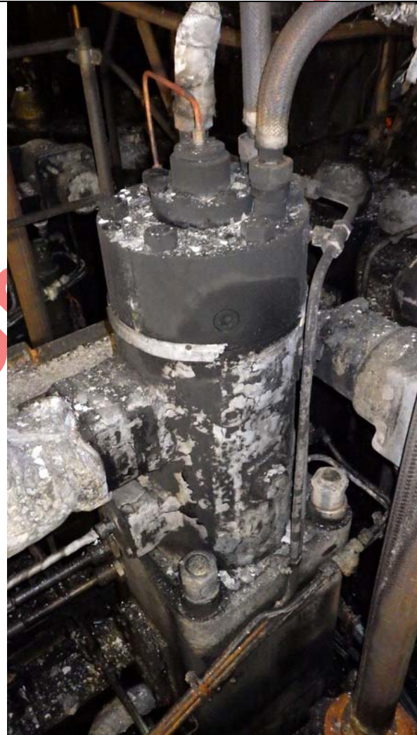
High pressure fuel pump, shock absorber, roller guide bush/housing. Condition unknown
