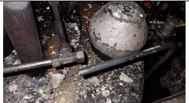
Return pipe for fuel valves disconnected/pulled out of fitting
