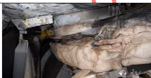
Turbocharger #2: Damaged insulation for gas inlet.
