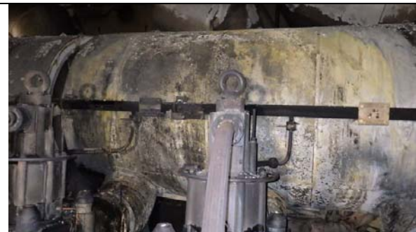
Exhaust gas receiver sheet metal and insulation damaged
