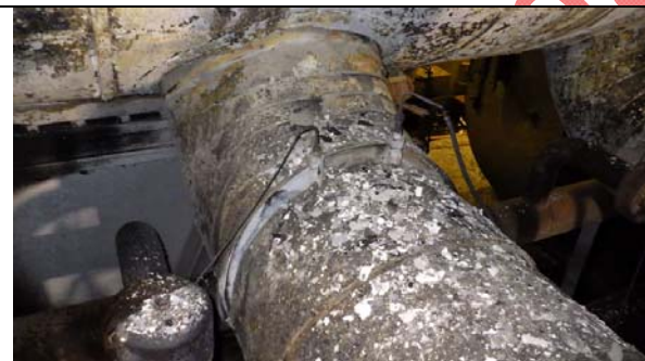
Exhaust valve compensator sheet metal and insulation damaged
