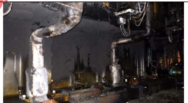
Cylinder frame cam side and underside of cam shaft housing exposed to heat from the fire. Damaged pipe insulation
