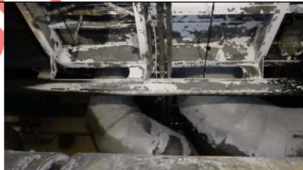
Deck above main engine and rail for engine room cranes damaged and deformed due to extreme heat exposure
