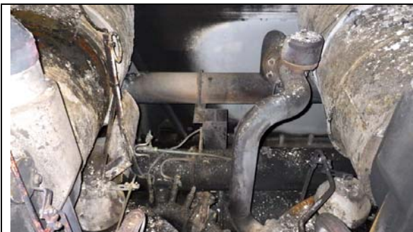
Start air pipe for start air valve and start air header pipe exposed to extreme heat
