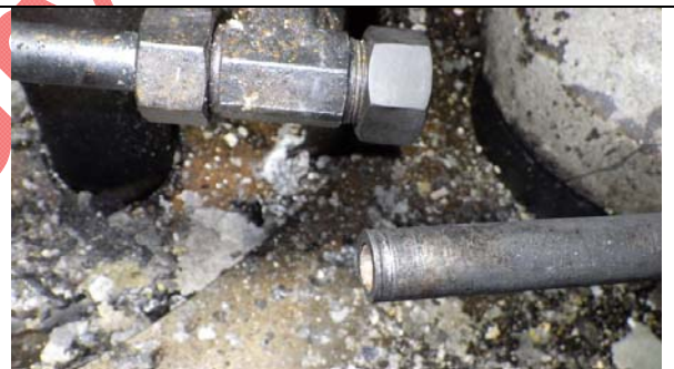
Pipe end pulled out of fitting
