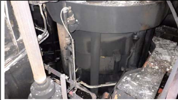
#6 Cylinder cover and cylinder liner. Condition unknown
