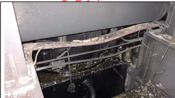
Cables and wiring on exhaust side damaged.
