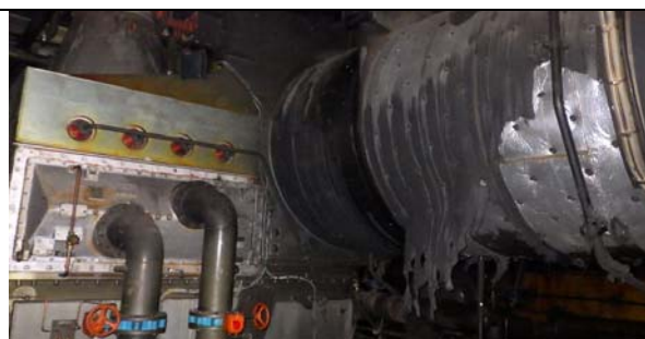
Damaged insulation for scavenge air receiver between air cooler #2 and #3
