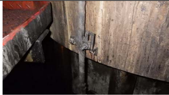
Return pipe for fuel valves correctly mounted with pipe hanger attached to cylinder cover.
