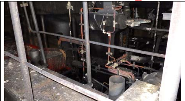
Damaged copper tubing cylinder unit #7
