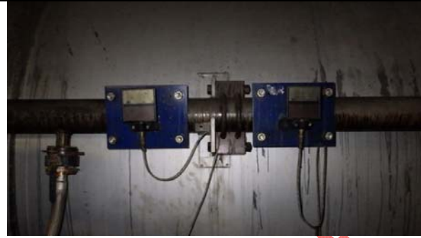
Cylinder unit monitoring instruments intact
