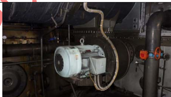
Example of electrical motors exposed to hot smoke an fumes.
