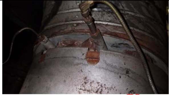
Sheet metal for exhaust valve compensator flange not seated correctly, exposing hot surface
