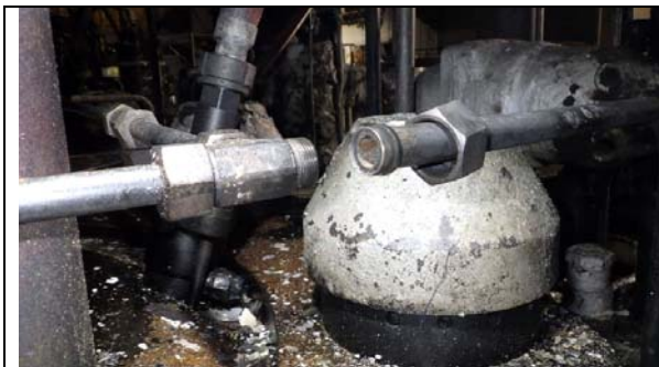
Ferrule not mounted correctly. (Ferrule and union nut mounted on pipe for example of explanation)
