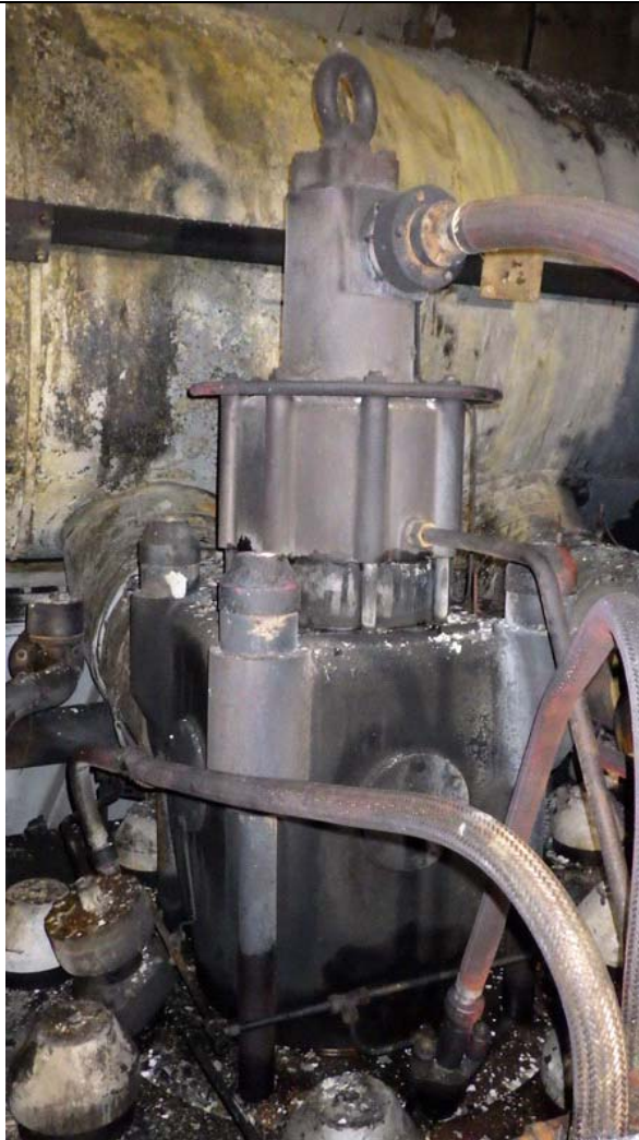
#5 cylinder unit: Exhaust valve, fuel valves, fuel valve high pressure pipes, starting air valve, cylinder cover. Condition unknown
