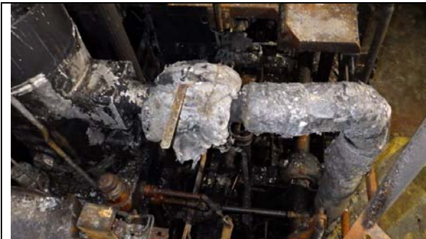
Fuel pump: Fuel supply pipe and insulation
