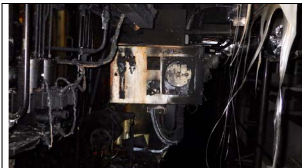
Damaged Emergency/Engine side stand and control panel instruments missing/melted
