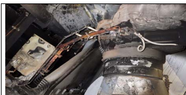
Damaged air cylinder and insulation for TCCO gas inlet. Turbocharger #2
