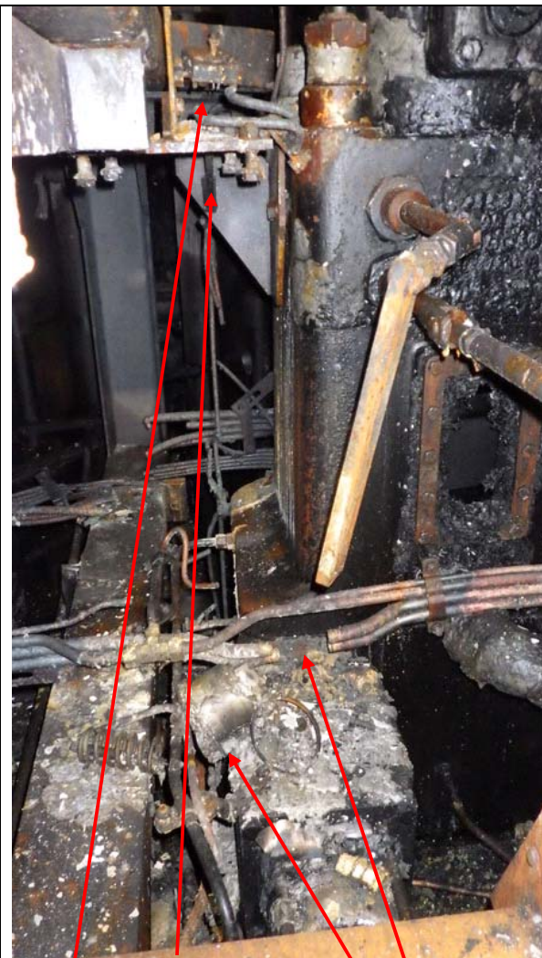
VIT Cylinder melted, remaining laying on top of housing for reversing mechanism. Device for lifting gear controlling melted. Copper tubing for control air sagging, brass fittings (T-pieces and straight male couplings melted)
