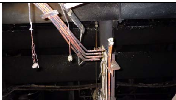
Damaged copper tubing and electrical wiring for turbo charger cut out.
