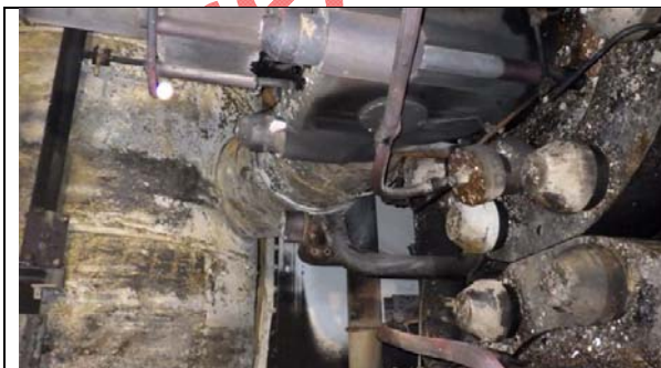
Fuel return pipe spraying on start air valve, exhaust gas receiver, exhaust valve compensator.
