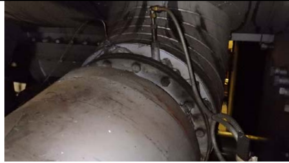
Sheet metal and insulation missing for exhaust valve compensator flange, exposing hot surface
