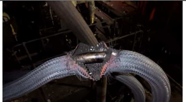
#6 fuel valve high pressure pipe "centre": Steel protective hose burst
