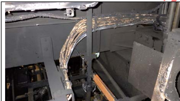
Damaged insulation on cables for engine control and monitoring.
