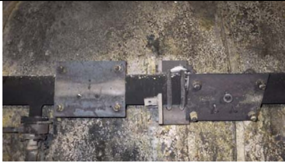
Cylinder unit monitoring instruments missing/melted
