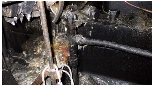
T-connection and non return valve for fuel return pipes from fuel valves and fuel pump.
